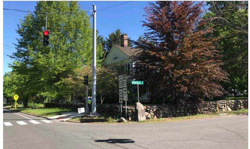
Accessible Drop Ramp without Sidewalk Connection at the Corner of RT 57 and Norfield Road
