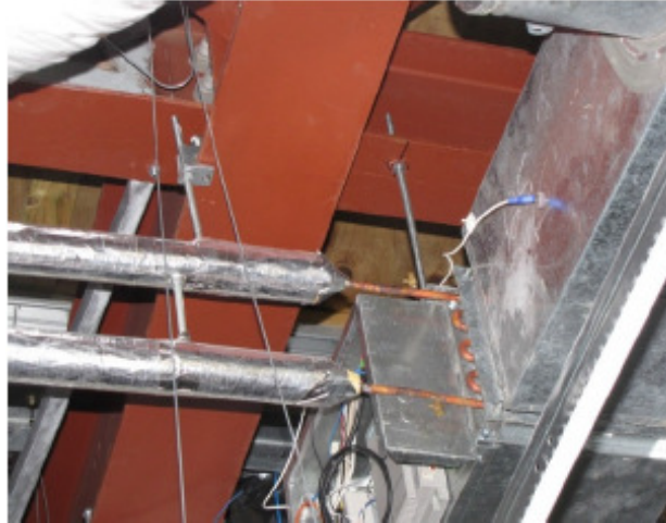
Figure 5: Lack of flexible connections to mechanical plant
