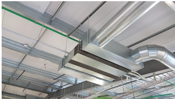
Figure 16: Non-compliant installation of overhead mechanical plant (no lateral restraint provided) – building completed and received Code Compliance Certificate 2015
