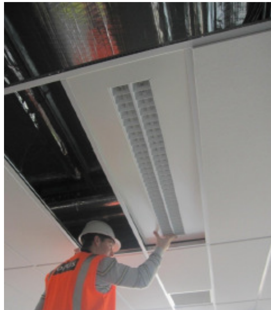
Figure 8: Unsecured recessed luminaires
