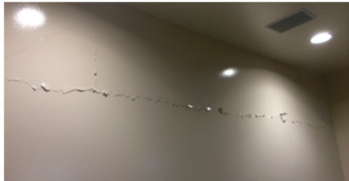
Figure 12: Cracked gypsum board wall in hospital
