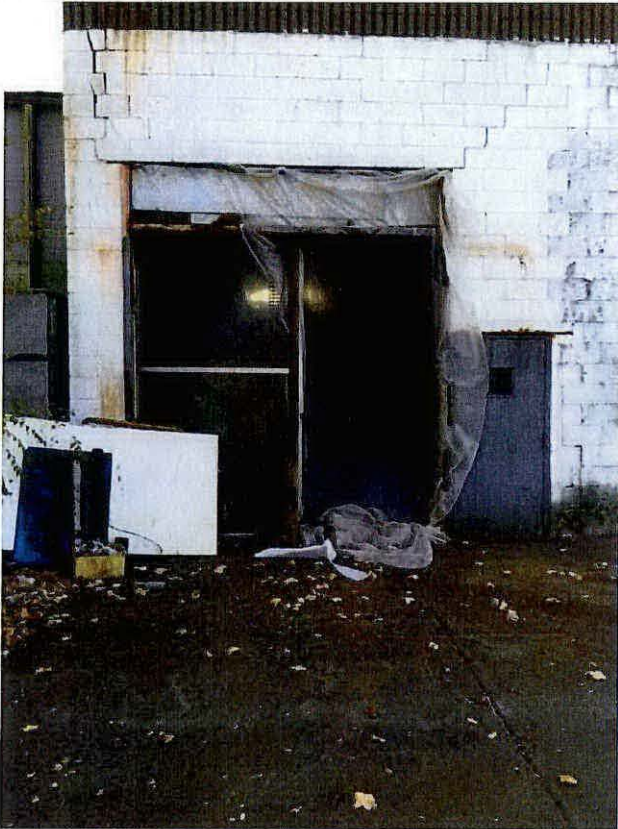
Photo 41: Missing bay door on north side of building
