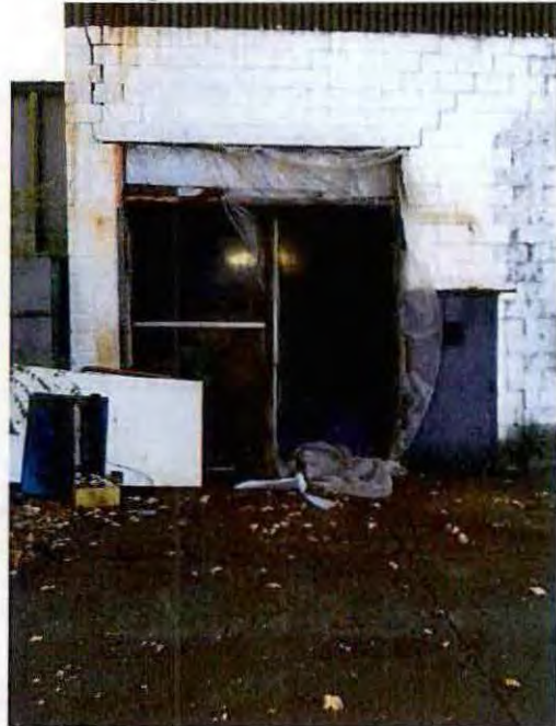
Photo 41: Missing bay door on north side of building
