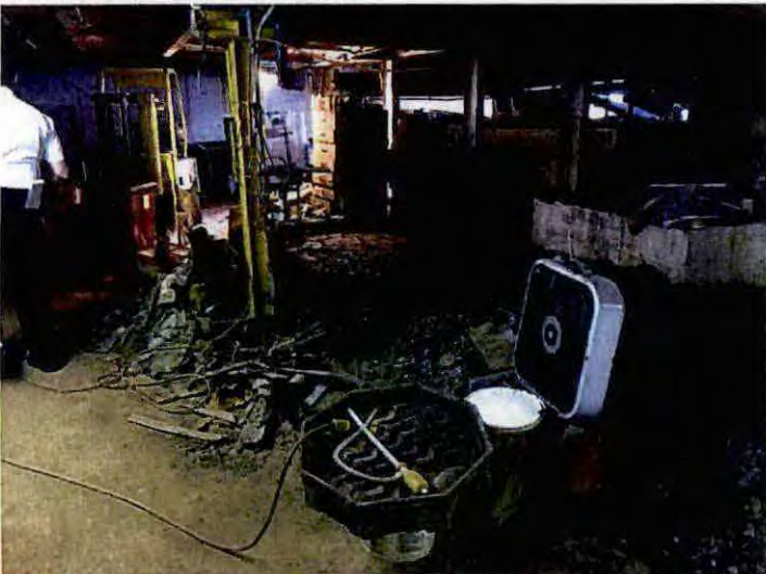
Photo 51: Sludge drying in basement. Note purported F006 listed hazardous waste used as berm material
