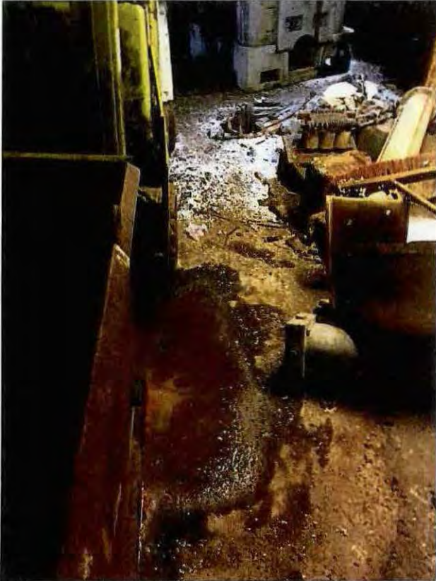
Photo 13: Pooled leakage in basement
