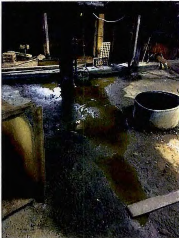
Photo 12: Pooled leakage in basement
