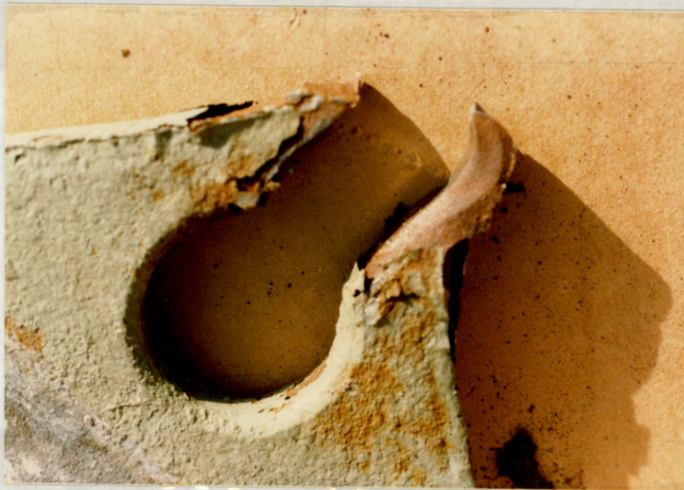
Figure 6. This Figure shows the failure of the eye in the plate when a shackle was pulled through it.
