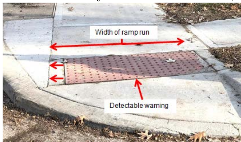
Exhibit 7. Detectable Warning Not Extended Across Full Width of Ramp
