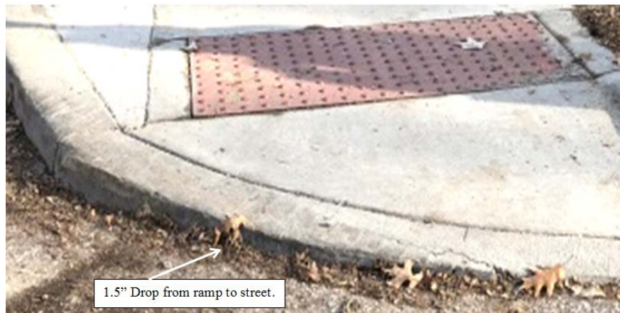
Exhibit 6. Curb Ramp Not Flush with Pavement
