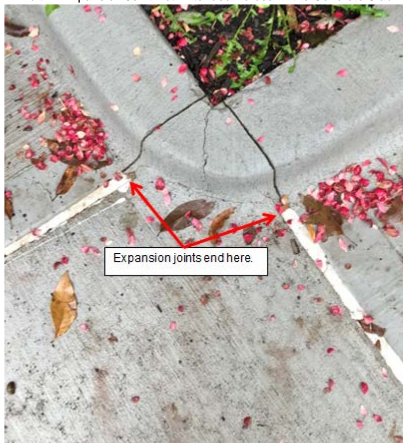
Exhibit 2. Expansion Joint Not Extended Across Entire Concrete Slab
