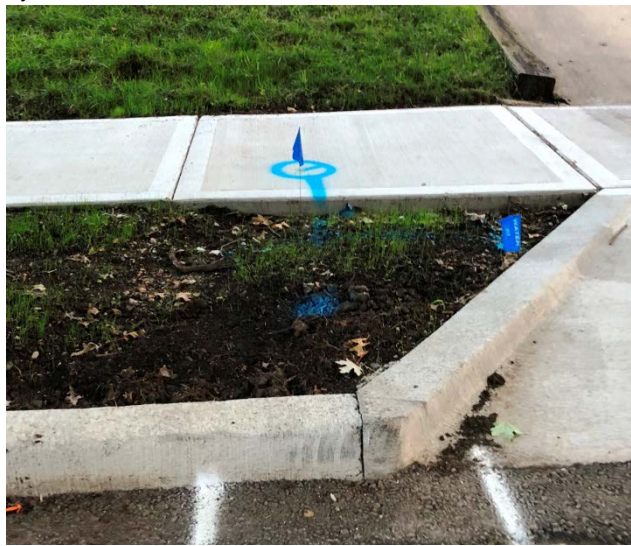
Exhibit 3. Curb Stop Box (Marked with Blue Circle) Covered by New Sidewalk
