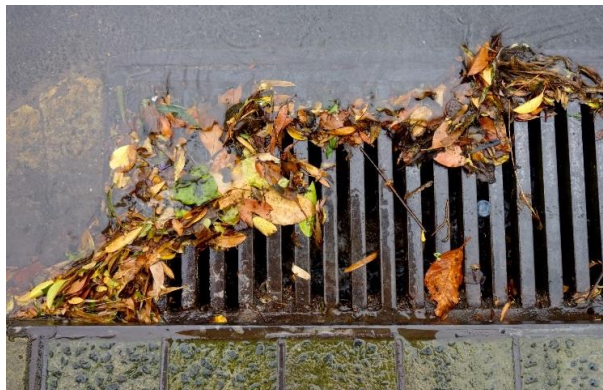
Figure 69 - Organic debris in storm drain
