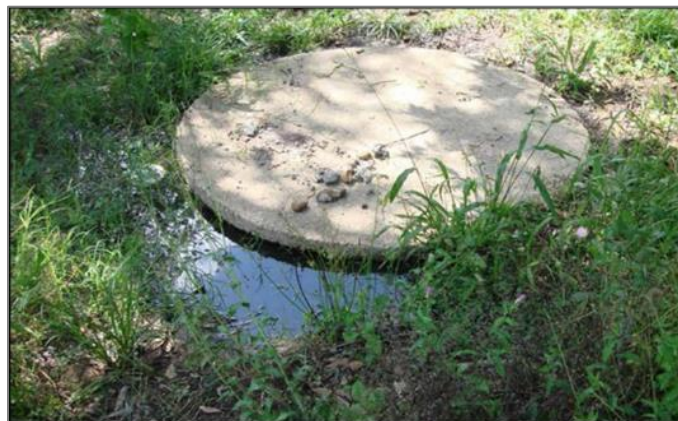
Figure 67 - Sewage from a failed septic tank 101
