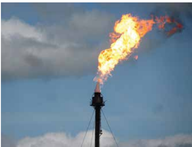
Petrochemical plants use flaring to consume waste gases by combusting them in an open flame.
