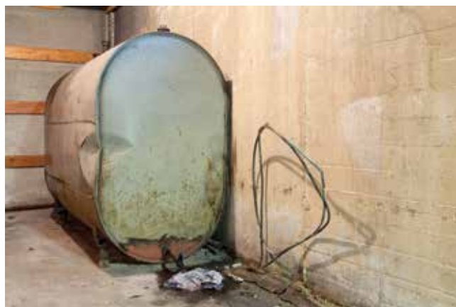
Example of a poorly maintained home heating oil tank in basement.
