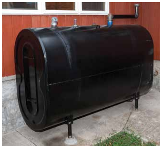
Example of outdoor above-grade fuel storage tank.
