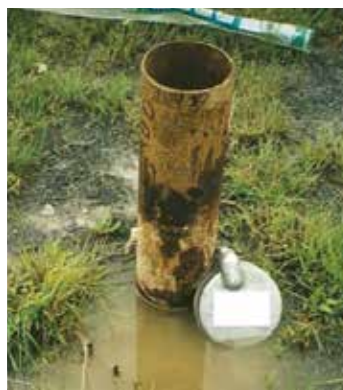
Poorly maintained water supply well.
