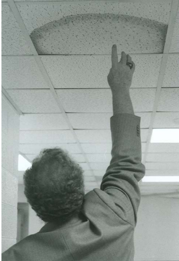
PDK auditor pointing out water damage in the hallway at Johnson Elementary School
