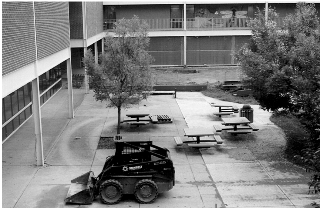
The high school was undergoing renovation as shown in this photograph at the time of the audit
