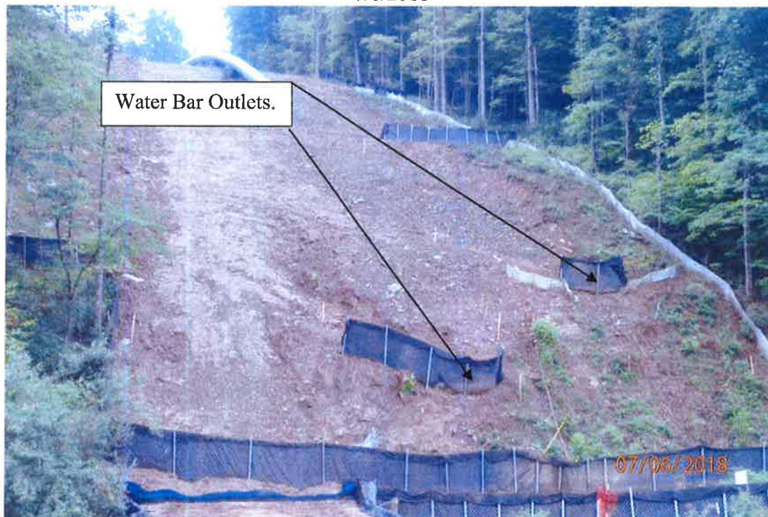
Water bars that are not installed properly and do not shed stormwater off of the LOD in small quantities as designed located adjacent to Laurel Run of Meathouse Fork crossing. Deficiencies in site evaluation item numbers 1, 7, 19 & 21 pictured.
