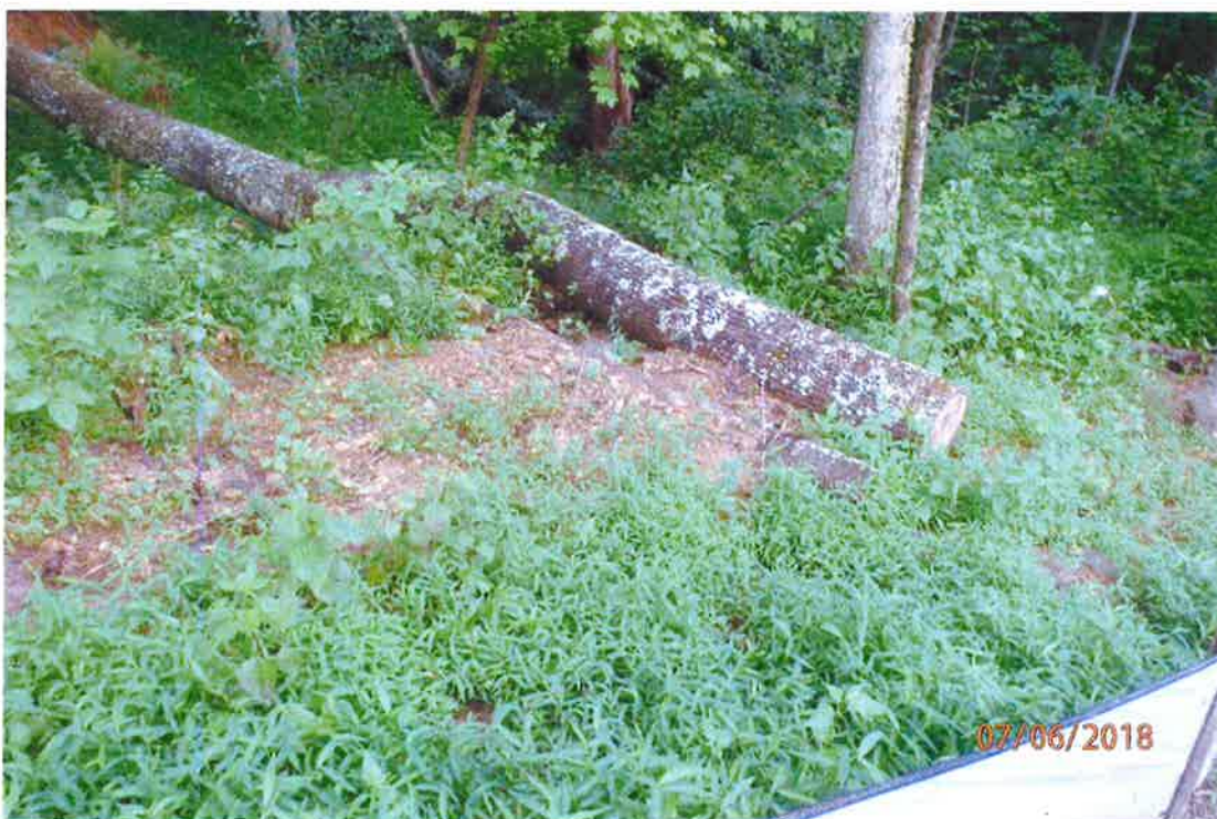
Water bar that has been installed at a steep angle with erosion and the associated offsite sediment deposits. Deficiencies in site evaluation item numbers 1, 7, 19 & 21 pictured.
