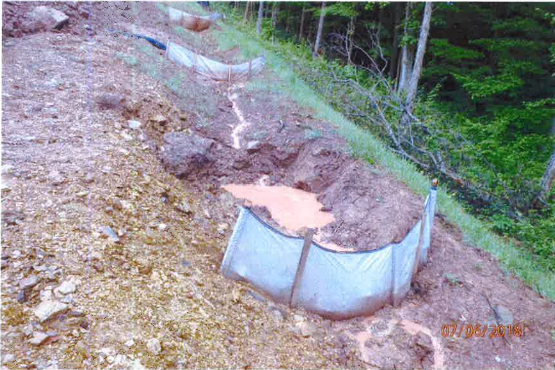
The installed temporary right of way diversion and outlet adjacent to 1851+00 that was collecting stormwater from multiple water bars and it did not have adequate outlets. This caused concentrated flow to overwhelm the installed BMP at the base of the slope. Deficiencies in site evaluation item numbers 2, 6, 7, 19, 20 & 21 pictured.
