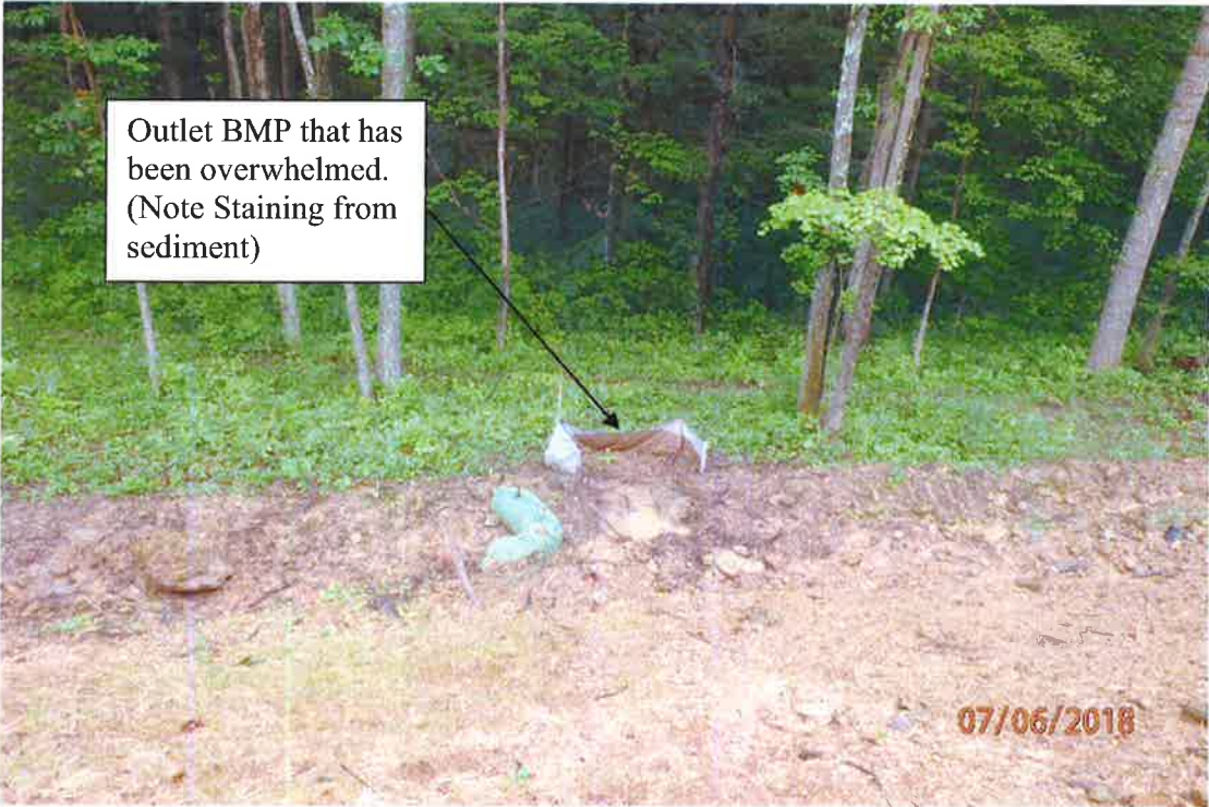
Installed temporary tight of way diversion and outlet that does not have adequate outlets adjacent to 1876+00. Evidence of the terminus BMP being overwhelmed in lower picture. Deficiencies in site evaluation item numbers 2, 6, 7, 19 & 21 pictured.
