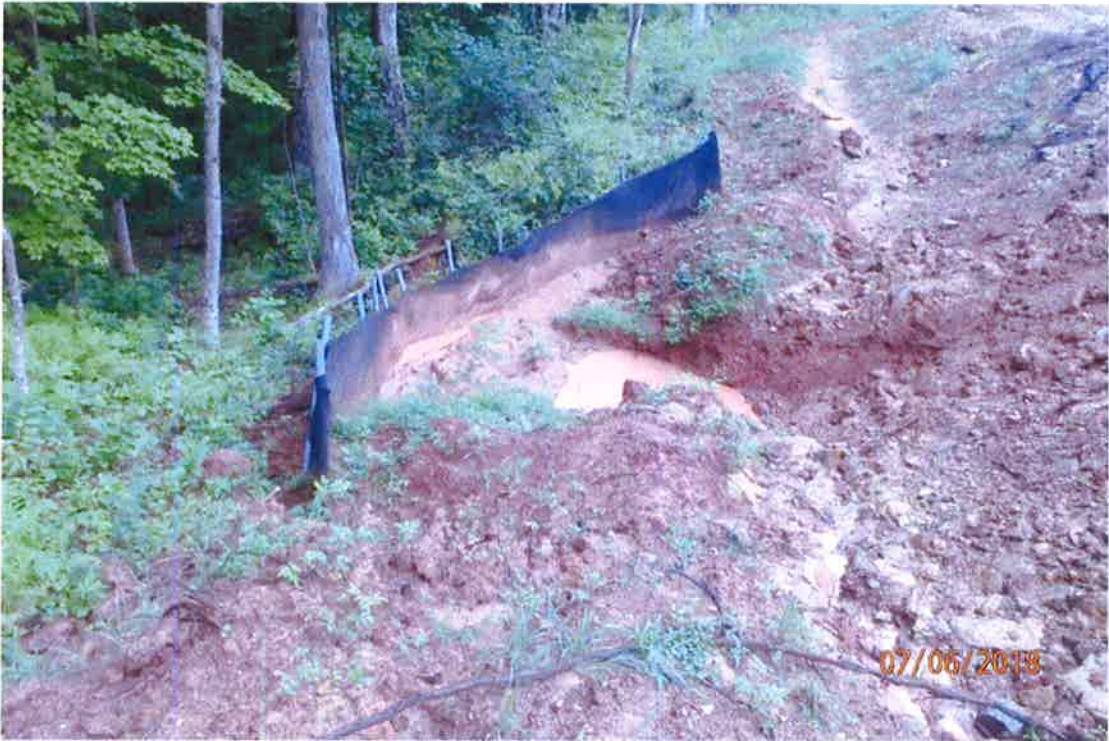
Overwhelmed BMP at the base of the slope adjacent to 1851+00.
