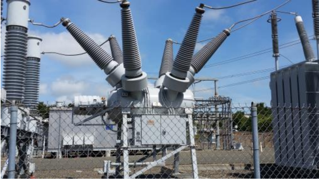
Figure 1: One of Valero Substation's breakers located within PG&E's Bahia Substation
