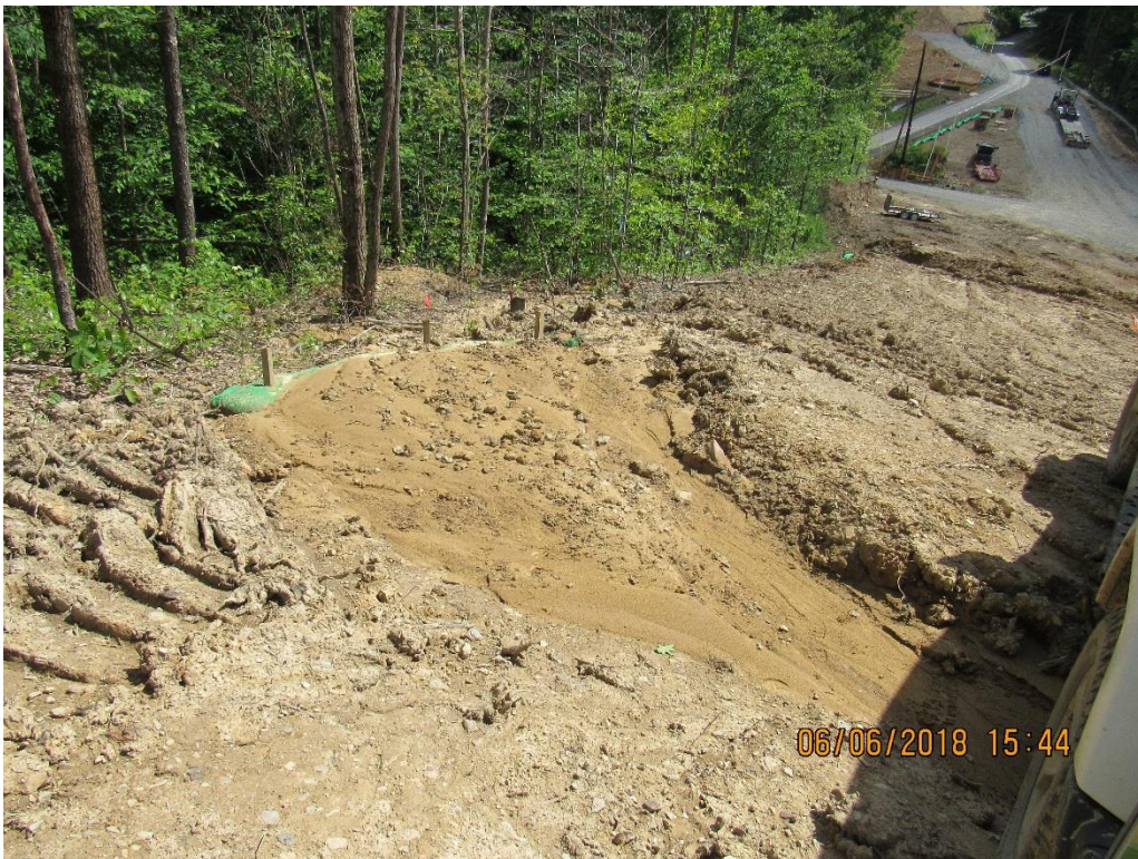
Photo 8: Control failure near station 6854+00 where sediment laden water left site.
