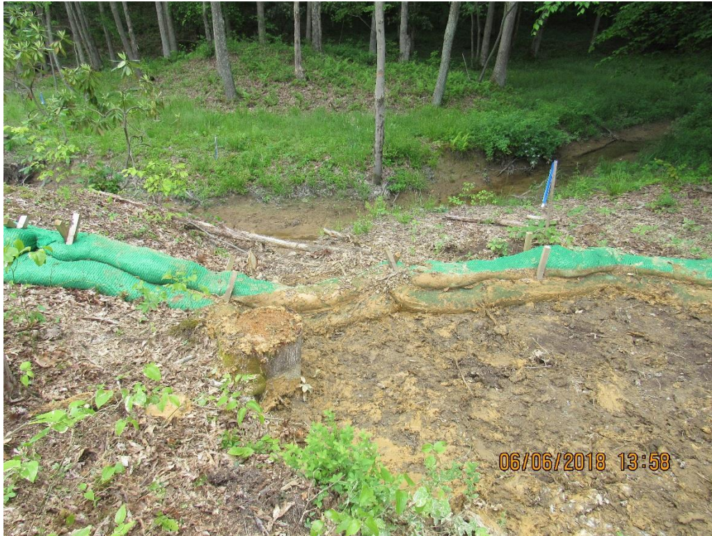
Photo 1: Station 6782+00 control failure repair but additional controls not added.
