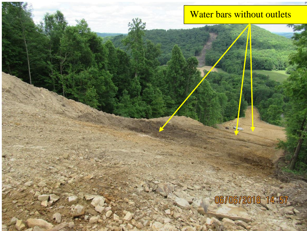
Photo 3: Water bars installed without adequate outlets near station # 6801+38 with <24^{\circ} to >30^{\circ} slope.
