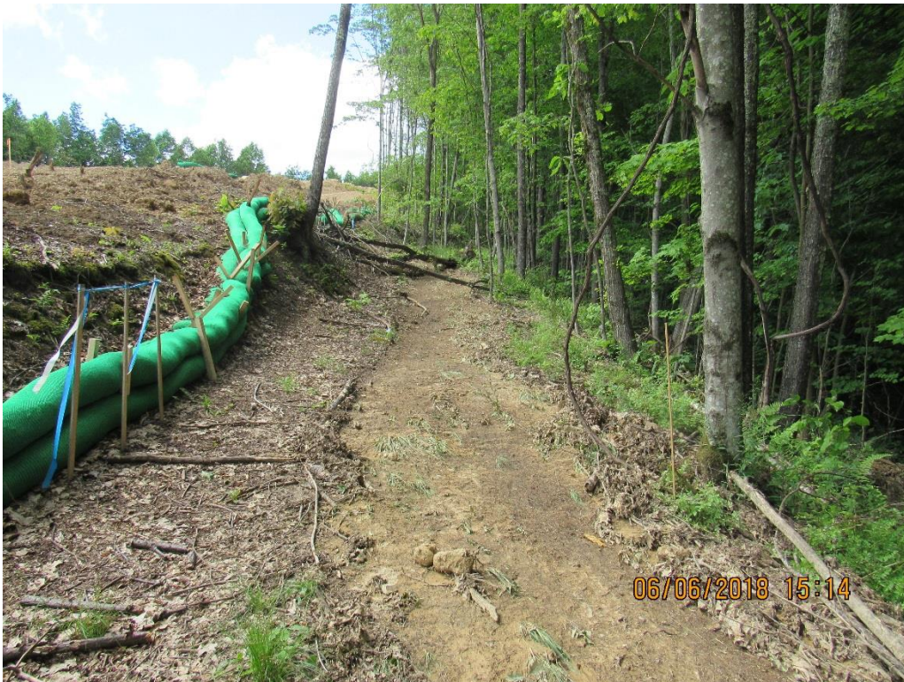
Photo 5: Scoured path from control failure at station 6812+58.
