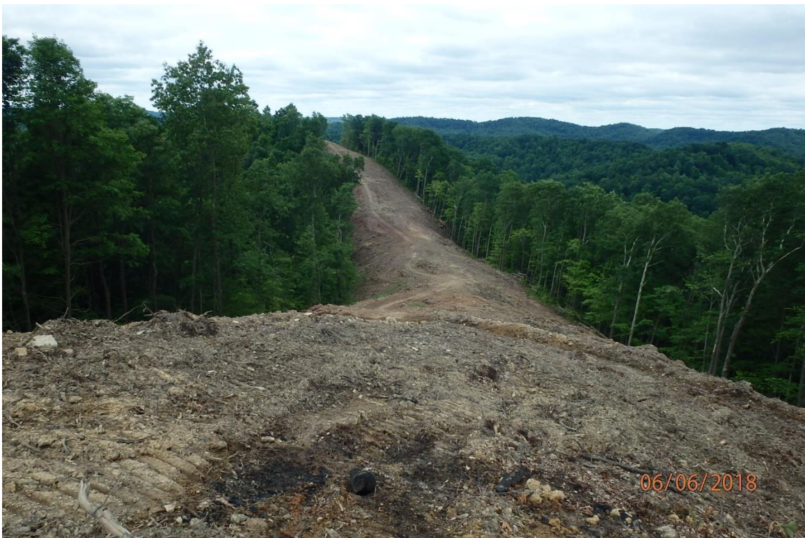
Areas of the project that have been cleared to mineral soil and BMPs are not in place as indicated in the SWPPP. Deficiencies in site evaluation item numbers 1, 7, 8, 13, 15, 19 & 21 pictured.
