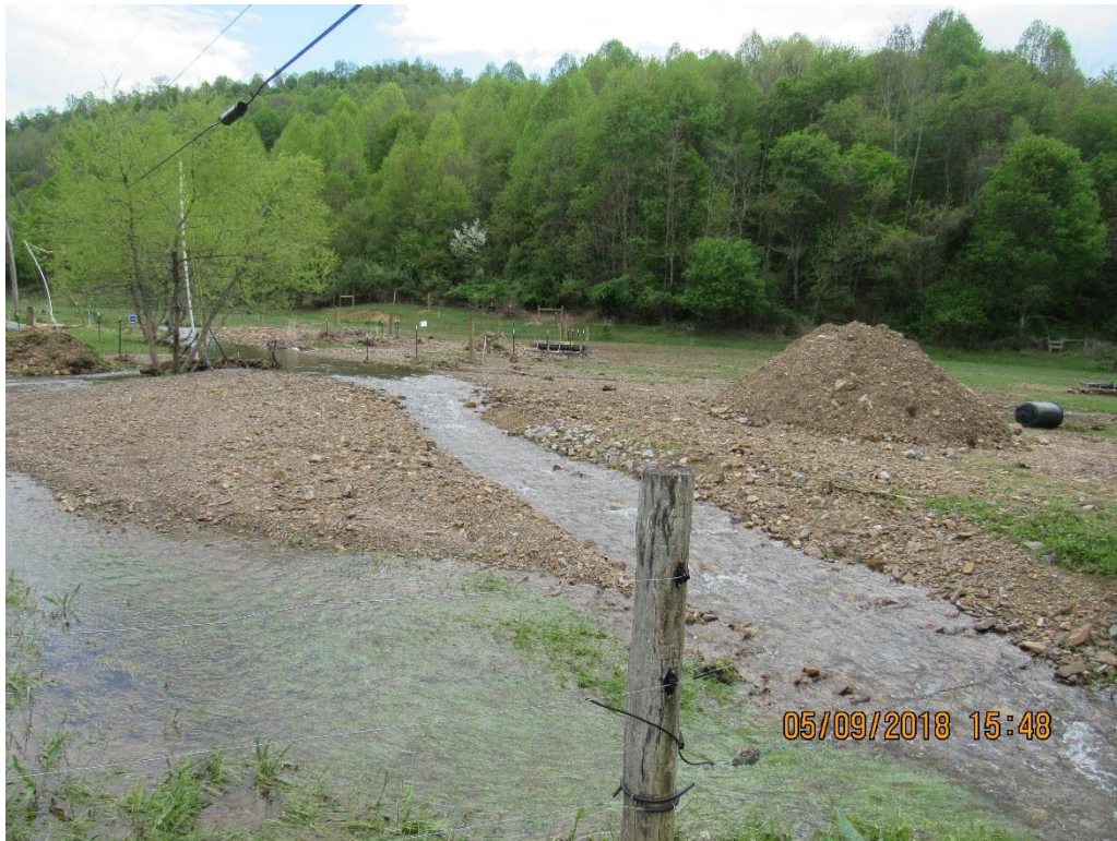
Photo 3: Mr. Laws field (station 10146+32, sheet 9.35)- stream has been partially returned to channel. Rock/soil pile from landowner removing debris to restore to channel.
