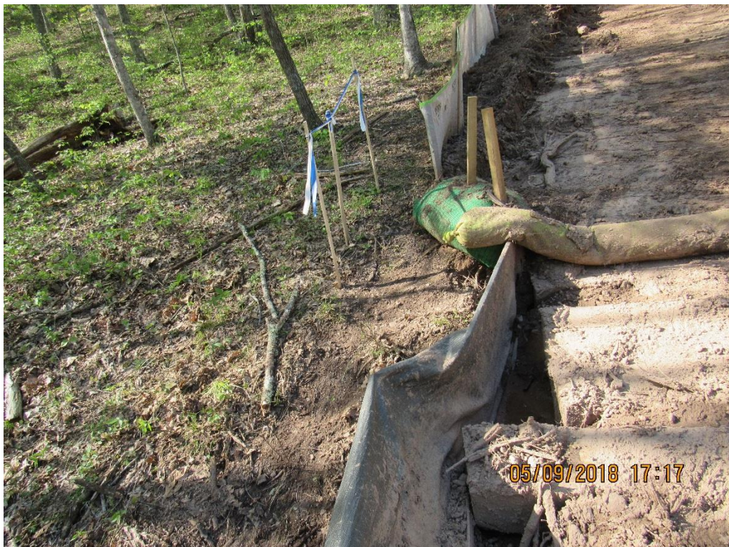
Photo 6: Location of control failure and breach allowing sediment laden water to leave site. Additional control (larger silt sock) added prior to bridge re-build.
