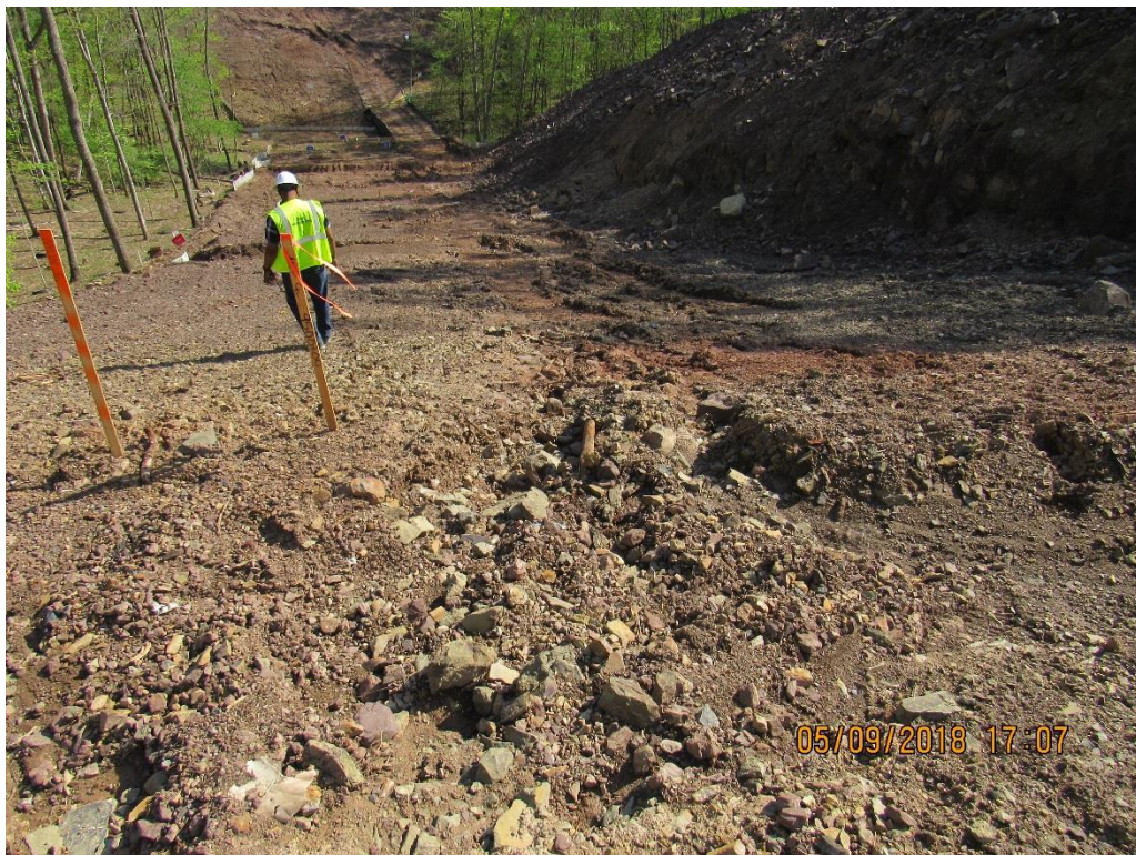
Photo 4: Downslope view of site of sediment laden water left site- erosion gullies observed on slope. (view south)
