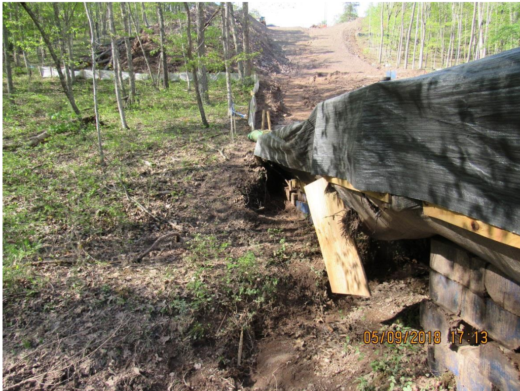
Photo 5: Stream crossing where sediment laden water left site after controls failed at stream S-IJ65 (view north). Additional controls added prior to re-building of bridge.
