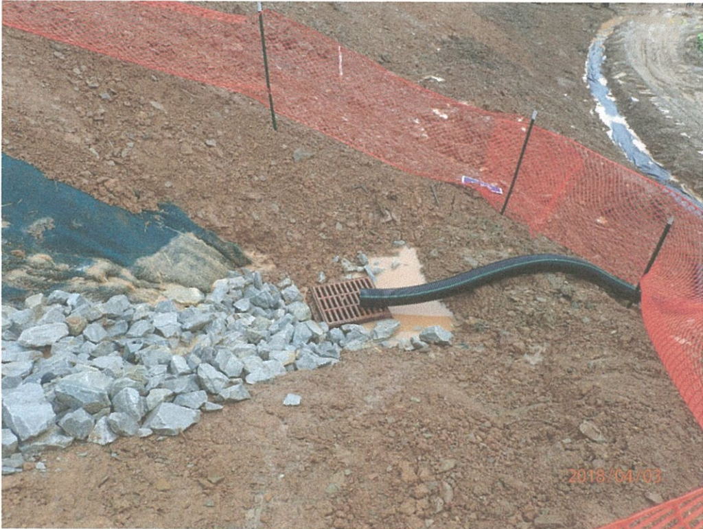
Unprotected drop inlet at Mobley Compressor Station.
