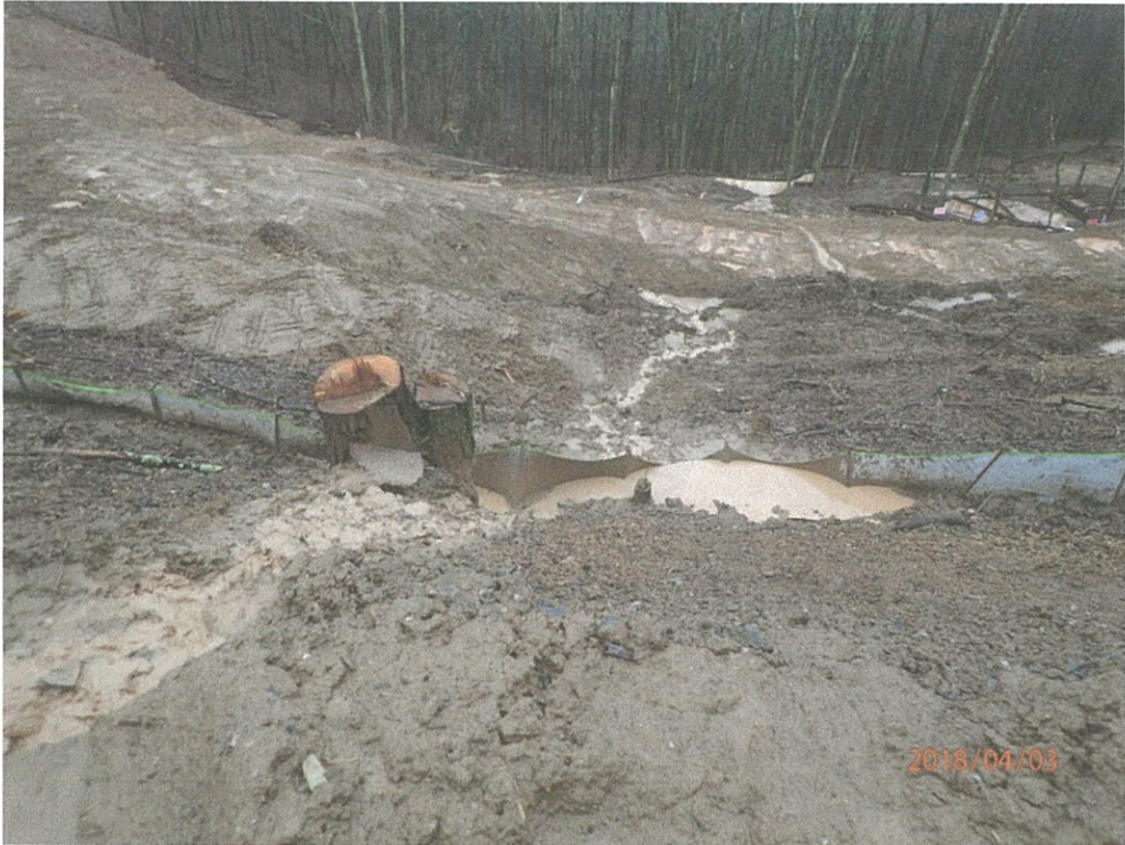
Concentrated flow eroding slope near slip.
