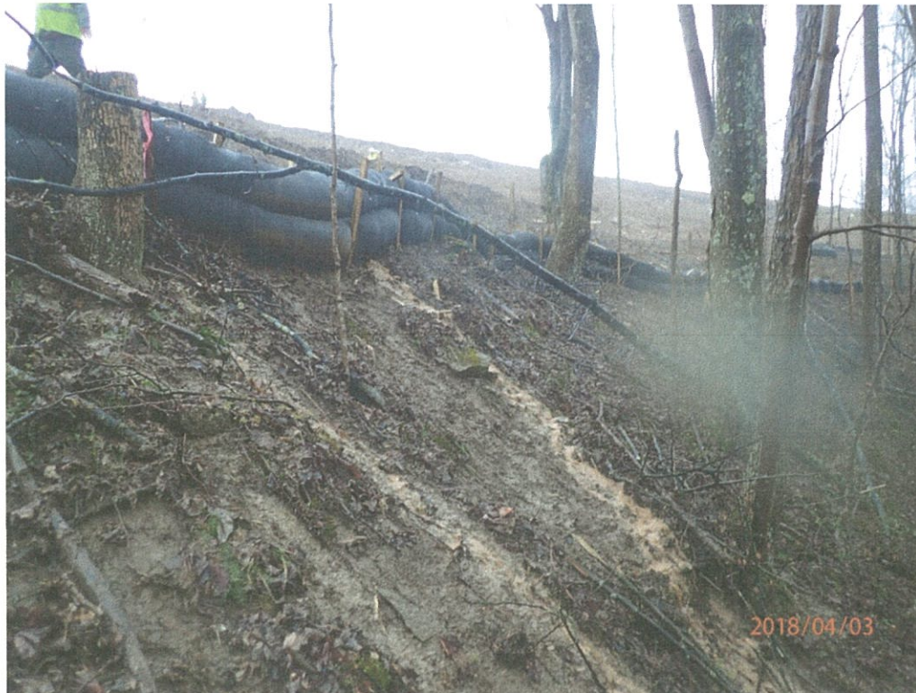
Sediment laden water leaving site at Bradshaw Compressor Station.
