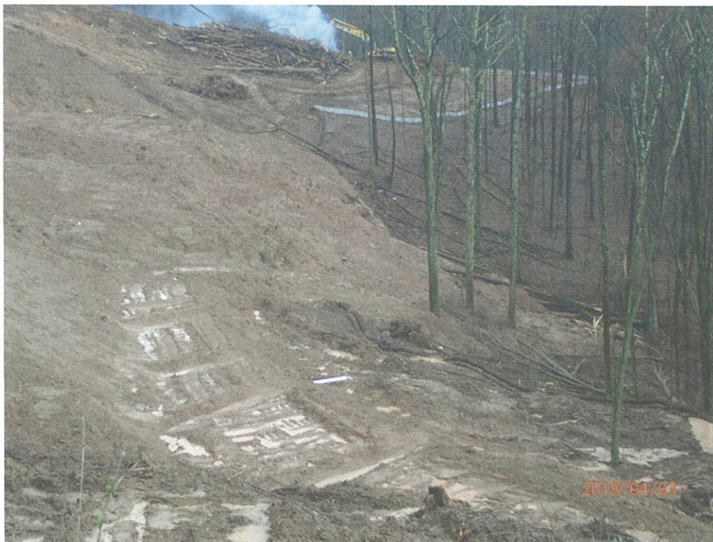
Reported slip area near Bradshaw Compressor Station.
