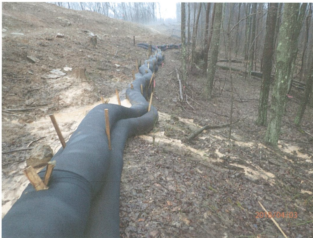
Second site of sediment laden water leaving site at Bradshaw Compressor Station.
