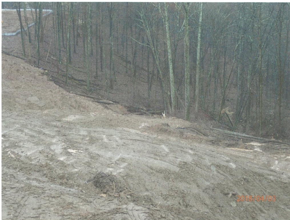
Slope above slip area.
