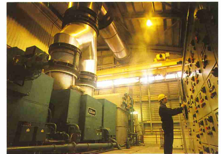
The fibropower power station at Eye in Suffolk, burns a dry mixture of poultry litter and wood shavings to generate electricity.
