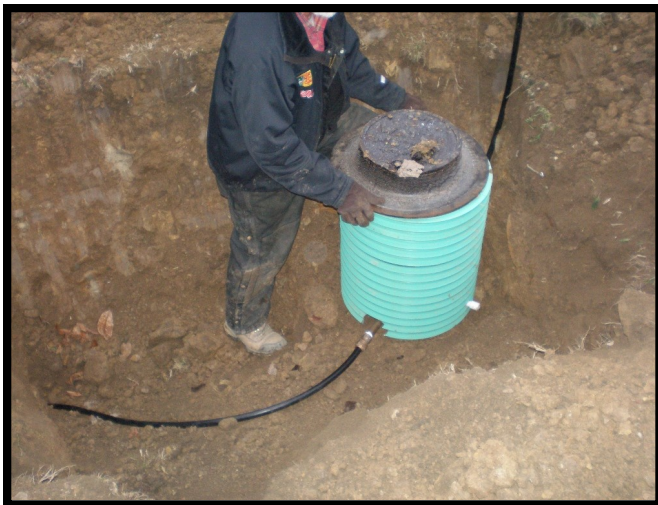
The metal lids on rural meters are often targeted.
