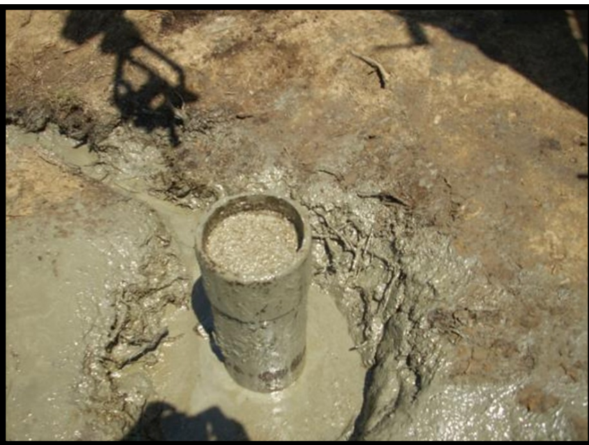
The plugging and abandonment operation of permit N17650 performed by Kirby Drilling.
