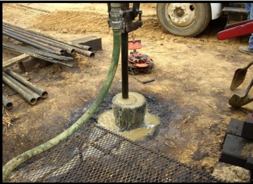
Class A cement displaced in casing of Permit N17650 (final stage of plugging), permanently plugging the well.
