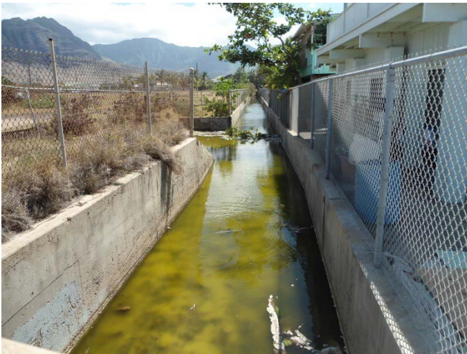
3. View of the City and County drainage canal along site southern boundary. View facing northeast.
