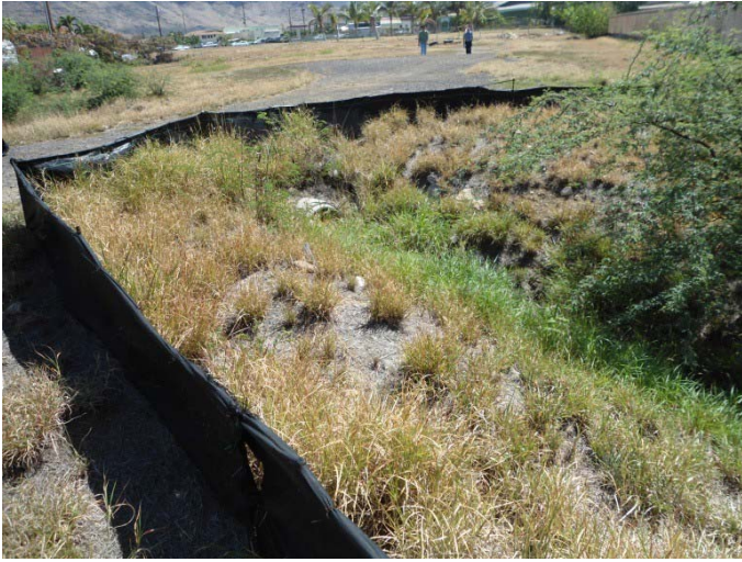
7. Drainage swale located in the southeast corner of the project site. View facing north.
