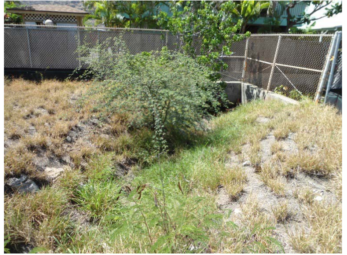
8. Drainage swale connecting to the City and County drainage canal. View facing south.
