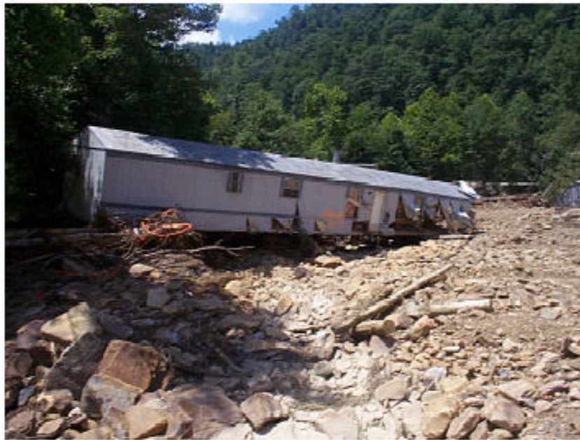
Figure L-2: Manufactured home damaged in floodway.
