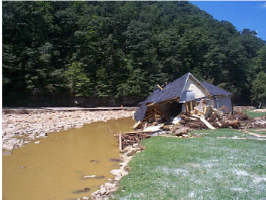
Figure L-1: Residential structure damaged in floodway.
