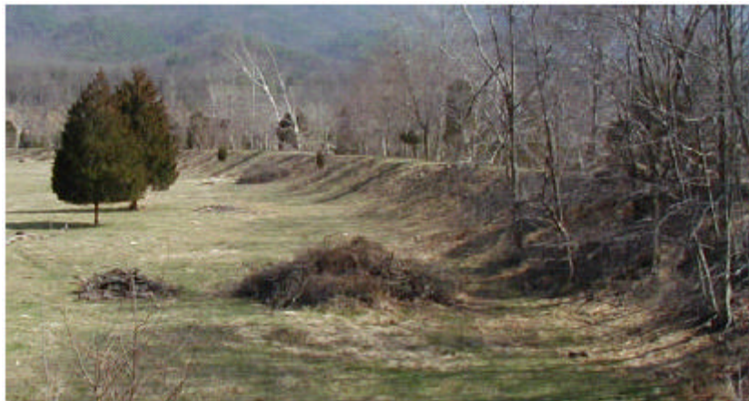
Figure H-4. Dredged Material Used To Construct An Un-Engineered Levee
