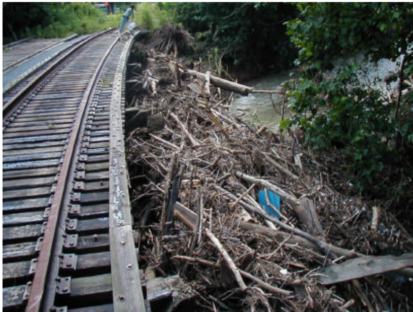
Figure F-8. Collection of debris at a railroad bridge.
