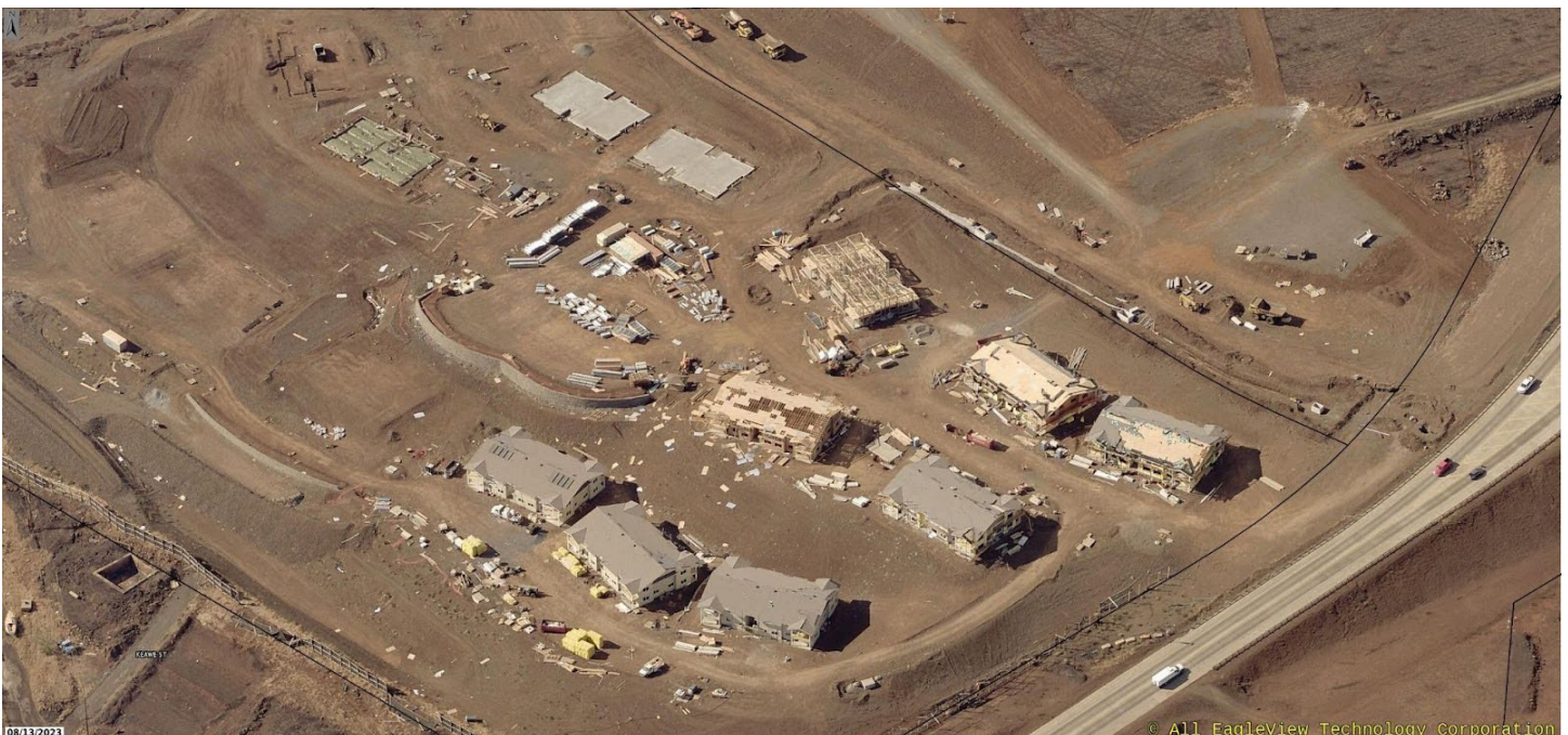
Figure 4.3.5.2.3 Wind damaged apartments at the construction site.
