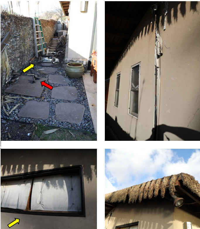
Figure 4.3.3.6.9 Close-up images of the structure at 1■ Kamaka Circle, showing that the extent of damage varied by multiple factors. Yellow arrow indicates the vinyl window frame that was impacted by radiant heat and fell out. Red arrow indicates ember ignition of wooden deck for what appears to be an outdoor shower.
