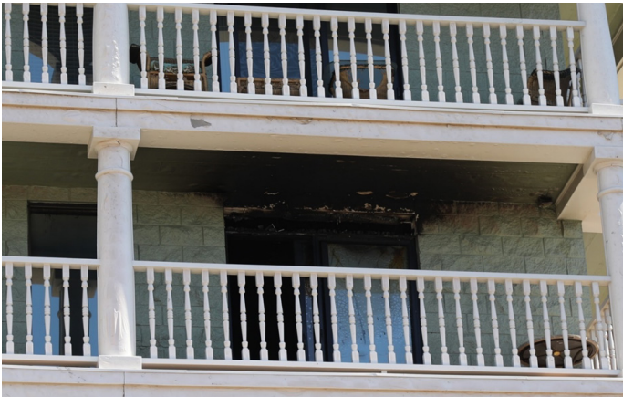
Figure 4.3.4.1.9 Close up of the open compartment on the fifth floor and thermal damage to furnishings on the sixth floor of 4 Front Street.
