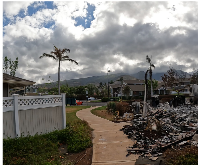
Figure 4.3.3.5.10 Photograph of space between Building 12 (shown on the right of the image) and Building 13 (shown on the left), showing minimal damage to the vinyl fence.
