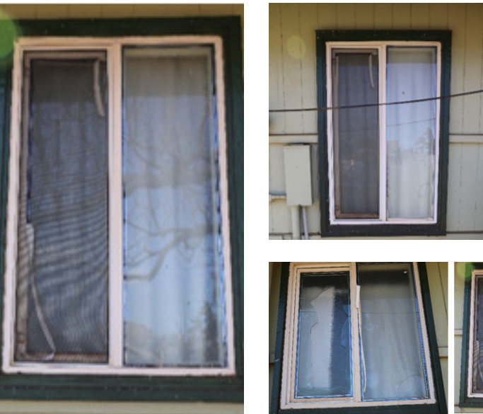
Figure 4.3.4.3.6 Window damage along the north wall of 3 Front Street.
