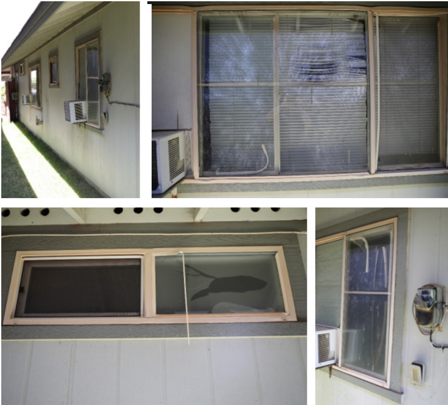
Figure 4.3.5.3.15 West side (makai) of 1█ 'Aipuni showing melted plastic components, damaged/broken window assemblies, and deformed window blinds likely caused by radiant heat transfer.
