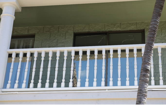
Figure 4.3.4.1.8 Close up of window damage on the second floor windows on the west (makai) room of 4 Front Street.
