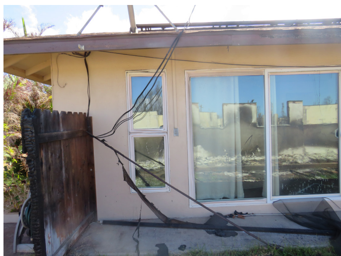
Figure 4.3.4.2.16 A wood fence connecting the west (makai) side of 6█ Kaua'ula to the wood fence on the 6█-5█ property line was destroyed up to the easternmost (mauka) panel that was connected to the structure. Had fire continued along this fence, it could have directly exposed wood eave structure and increased heat flux to the already damaged window immediately south of the fence.
