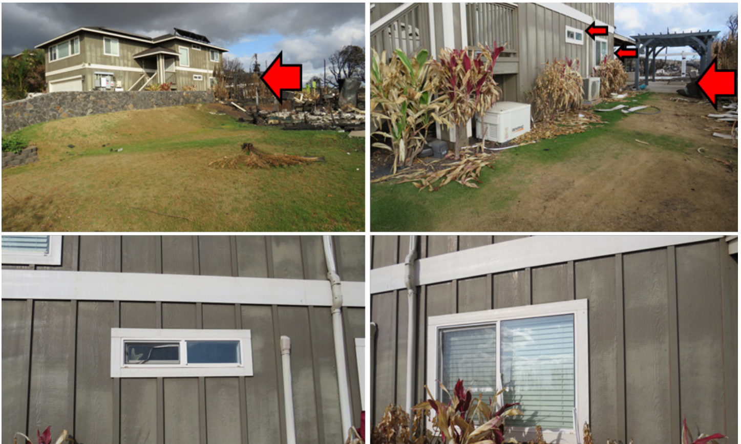
Figure 4.3.3.3.3 Damage classification assessment map to 3█ Komo Mai Street from (destroyed) 3█ Komo Mai Street; approximately 24 foot separation distance. Top left image shows both addresses, top right indicates the radiant heat vector in the generally opposite direction of fire spread. Bottom images show discoloration of fiber cement siding and deformation of vinyl window frames.
