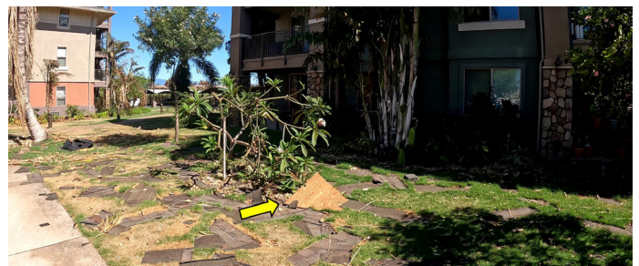
Figure 4.3.3.4.5 Wind damage to undestroyed apartment buildings, including significant roof covering (composition shingle) loss and roof sheathing.
