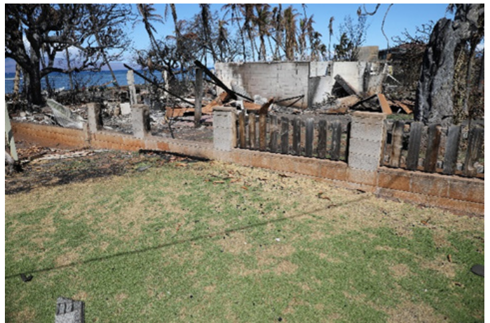
Figure 4.3.4.3.7 Burnt, charred, and broken wooden fence from the 3-3 Front Street property line directly connected to the structure at 3 Front Street. Wooden fences can act as a “wick,” carrying fire from one structure to the next. The northernmost panel was disconnected from the rest of the fence, removing this mechanism of fire spread.
