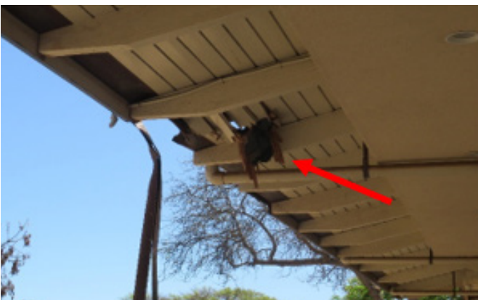
Figure 4.3.4.1.4 Utility pole south of Mill Street that hit and damaged the roof of the Boys & Girls Clubs of Maui.
