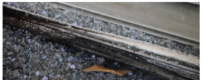
Figure 4.3.4.1.18 Destroyed chair proximate to rear patio door/window assembly on 4 Front Street, where the outer pane failed and inner pane remained intact. Note the indications of tempered glass in this assembly.
