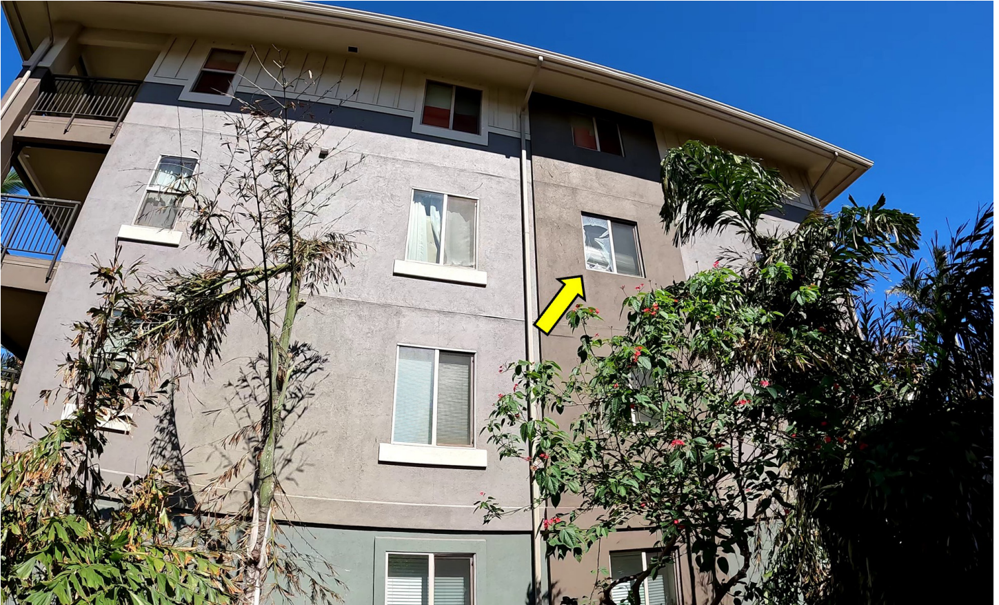
Figure 4.3.3.4.6 Broken window on third floor of eastern (mauka) side of apartment building, likely caused by windborne debris.
