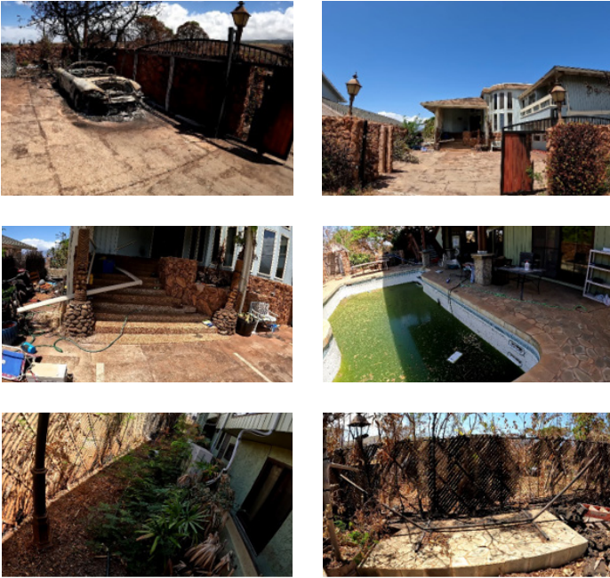
Figure 4.3.5.3.13 The 15███ Lokia Street lot experienced fire damage to the front entrance gate and destroyed a vehicle, but did not extend to the structure (top). The structure appears to have been defended, in part, by pumping water from the pool in the rear of the structure, powered by a battery system (middle). Damage to fences on the north and south sides of the properties (bottom), showing the end of the hose from the pump in the pool and along with a bucket (bottom left).
