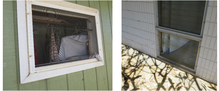
Figure 4.3.4.2.20 Examples of open/broken windows and/or screens in this cluster of surviving homes.
