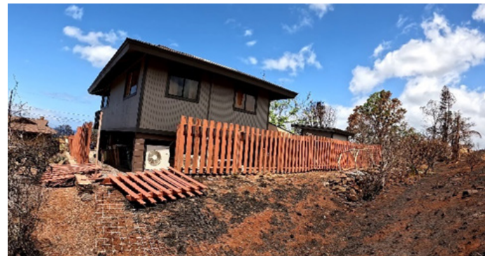
Figure 4.3.5.3.5 The surviving accessory structure at 16███ Lokia Street was near the eastern (mauka) property line, but was buffered from the grassland by a garden (note intact hoses and stone landscaping separating from the grass) and a fence. The structure was elevated such that the damaged windows were a longer distance from the burning vegetation than a single-story structure. Charred sections of fence were broken away from the posts and burning was stopped. Broken windows were boarded up from the inside by the time images were collected.
