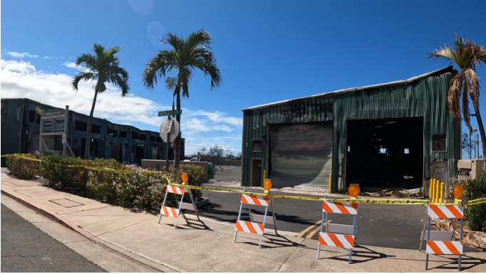
Figure 4.3.5.1.20 Emerald Plaza Building A consumed by fire.
