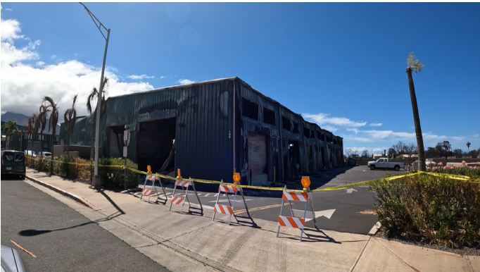
Figure 4.3.5.1.21 Emerald Plaza Building B and C consumed by fire.
