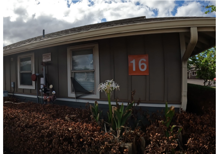
Figure 4.3.3.4.11 Thermal damage (window) to the front of Building 16, across from Building 15 (destroyed).
