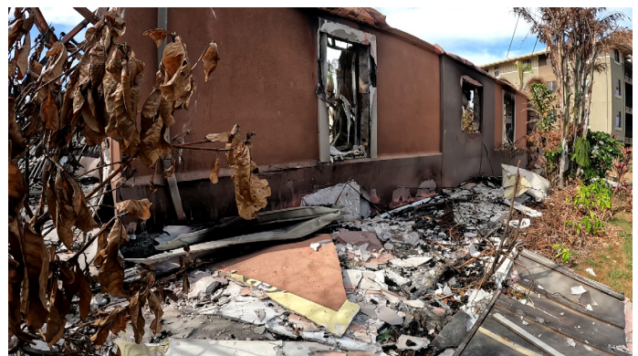
Figure 4.3.3.4.4 Destroyed apartment building showing CMU block exterior wall construction (first floor) and noncombustible sheathing with stucco finish coat and fiber cement siding.
