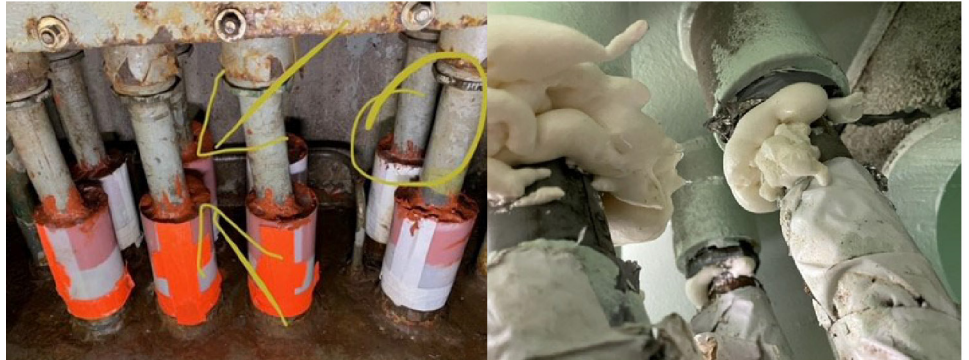
Figure 11: Use of Unauthorized Interventions, Including as Seen on Television Sealant Product and Plastic Wrap (left), Expanding Foam, Tape, and Common Store Bought Super Glue (right) as Documented by the Navy
