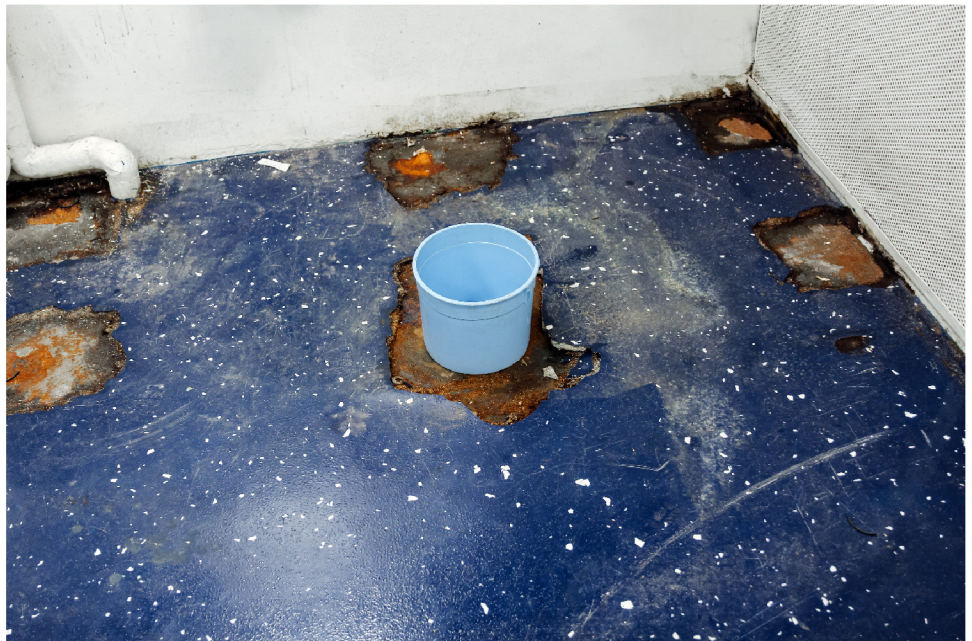
Figure 6: USS Cowpens Flooring Nearly 8 Years into Modernization
