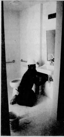
ACCESSIBLE: A workman installs a sink that can be reached by people who use a wheelchair.
