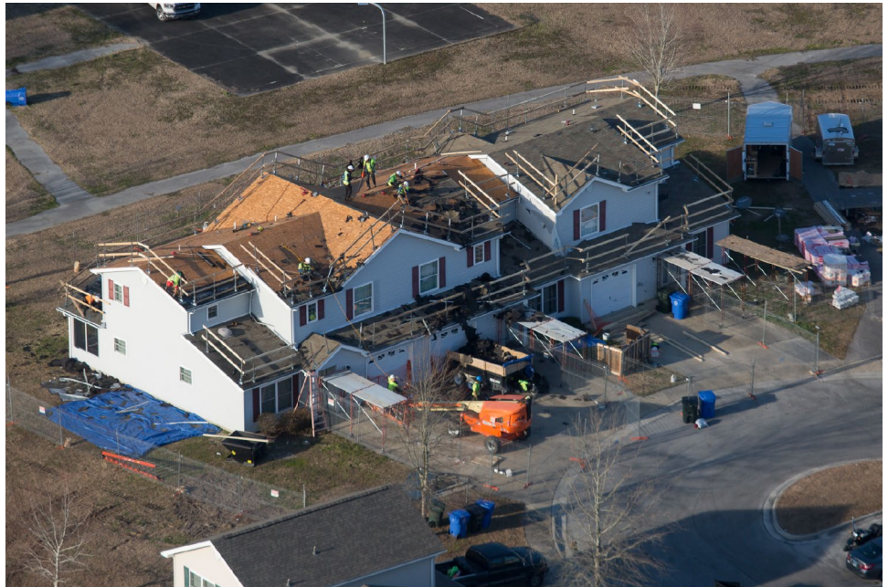
Figure 3: Significant Roof Repair to On-Base Privatized Homes at Camp Lejeune after Hurricane Damage
