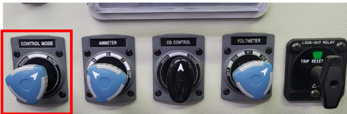
Step-down transformer controls, with the Auto/Manual Control Mode selector at far left. This photograph was taken post-accident.
