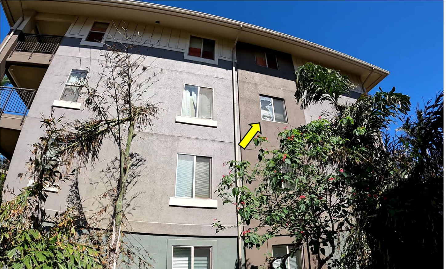
Figure 4.3.3.4.6 Broken window on third floor of eastern (mauka) side of apartment building, likely caused by windborne debris.
