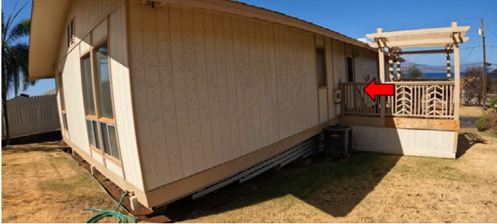
Figure 4.3.5.2.12 Northeast corner of 12█ 'Ainakea Road with blistering paint from radiant heat exposure (indicated by red arrow).
