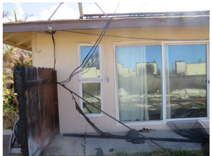
Figure 4.3.4.2.16 A wood fence connecting the west (makai) side of 6█ Kaua'ula to the wood fence on the 6█-5█ property line was destroyed up to the easternmost (mauka) panel that was connected to the structure. Had fire continued along this fence, it could have directly exposed wood eave structure and increased heat flux to the already damaged window immediately south of the fence.
