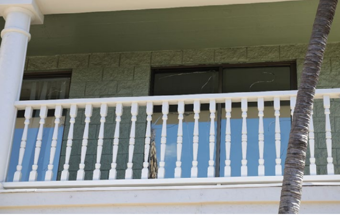
Figure 4.3.4.1.8 Close up of window damage on the second floor windows on the west (makai) room of 4 Front Street.
