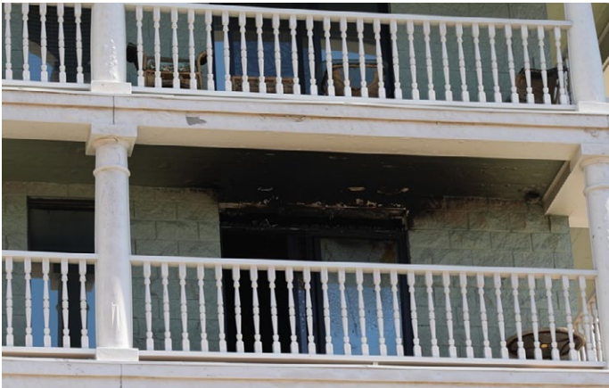
Figure 4.3.4.1.9 Close up of the open compartment on the fifth floor and thermal damage to furnishings on the sixth floor of 4 Front Street.
