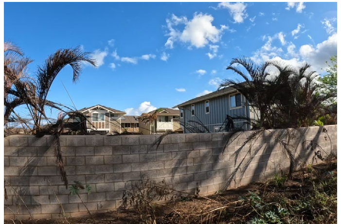
Figure 4.3.3.5.6 Destroyed single family home from the rear on the other side of the concrete wall.
