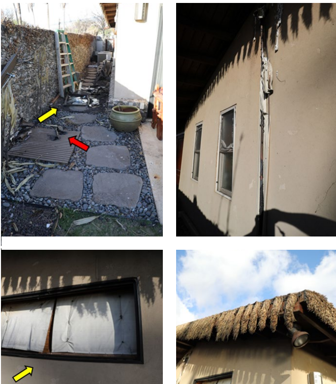
Figure 4.3.3.6.9 Close-up images of the structure at 1■ Kamaka Circle, showing that the extent of damage varied by multiple factors. Yellow arrow indicates the vinyl window frame that was impacted by radiant heat and fell out. Red arrow indicates ember ignition of wooden deck for what appears to be an outdoor shower.
