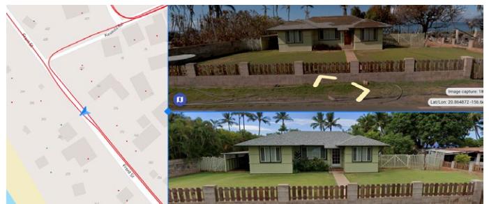
Figure 4.3.4.3.3 Strong winds removed shingles and tar paper from the roof of 3█ Front Street (top) and deposited much of this material in the west (makai) rear yard (middle).
