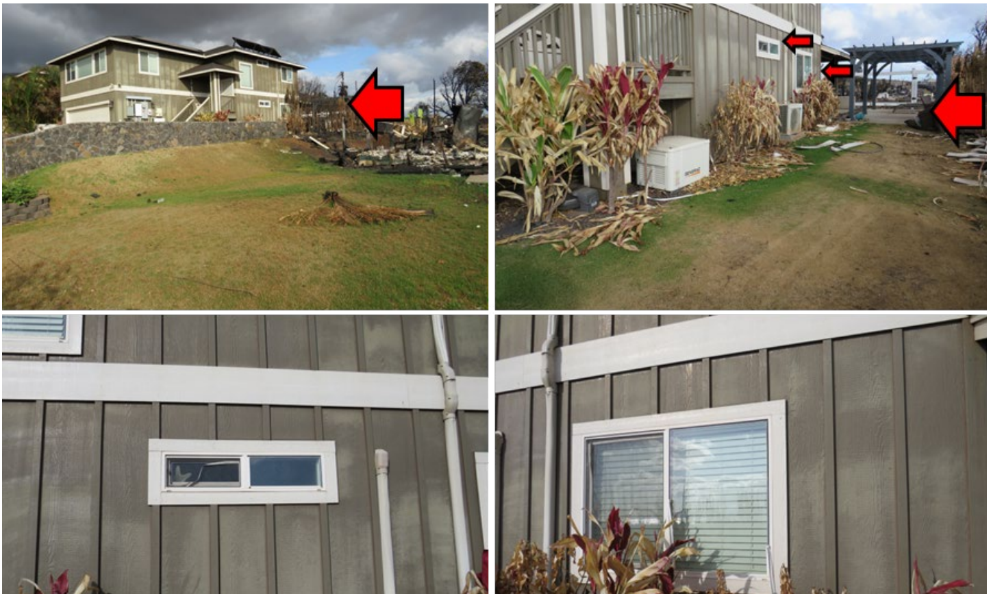
Figure 4.3.3.3.3 Damage classification assessment map to 3█ Komo Mai Street from (destroyed) 3█ Komo Mai Street; approximately 24 foot separation distance. Top left image shows both addresses, top right indicates the radiant heat vector in the generally opposite direction of fire spread. Bottom images show discoloration of fiber cement siding and deformation of vinyl window frames.
