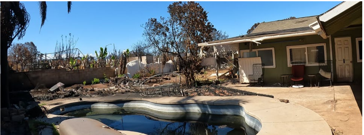
Figure 4.3.4.2.13 Exterior fire in the south yard of 7 Kāua'ula Road destroyed outdoor furnishings and structures up to the corner of the main residential structure. However, these fires did not spread to the south of the residence and appeared to result only in damage to the plastic gutter in the southwest corner.
