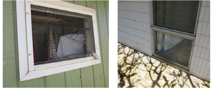
Figure 4.3.4.2.20 Examples of open/broken windows and/or screens in this cluster of surviving homes.
