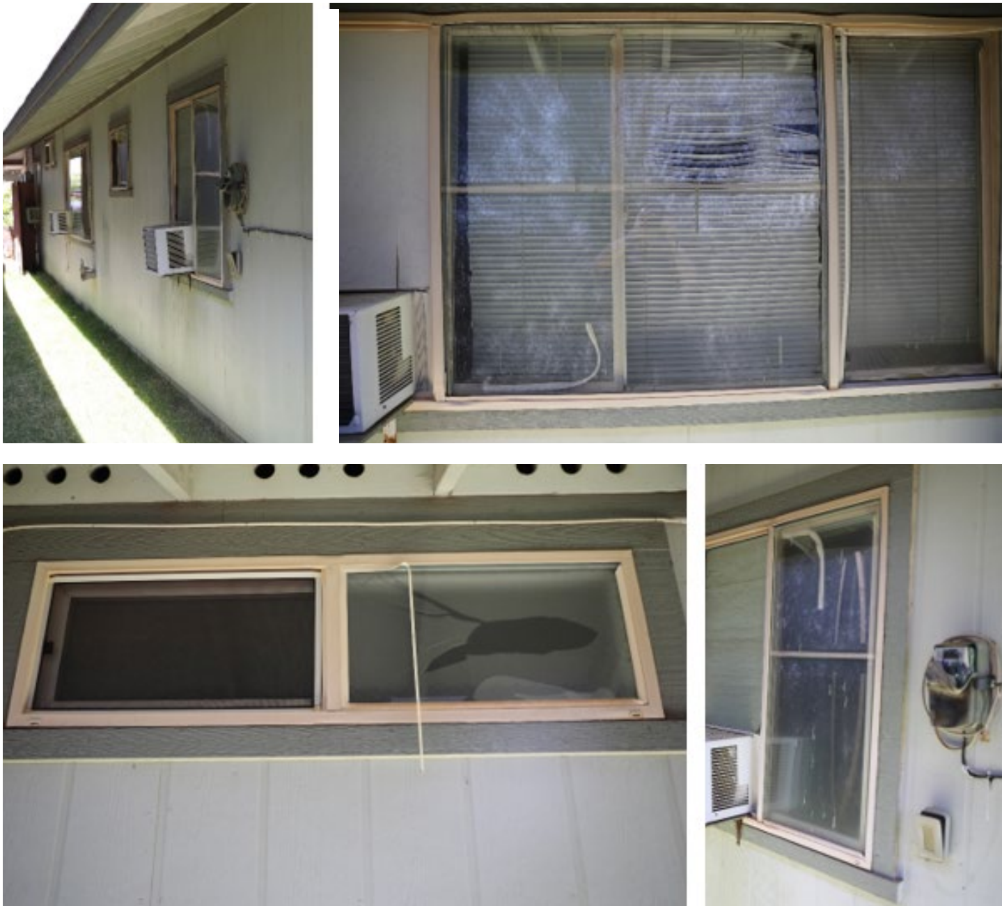
Figure 4.3.5.3.15 West side (makai) of 1█ 'Aipuni showing melted plastic components, damaged/broken window assemblies, and deformed window blinds likely caused by radiant heat transfer.
