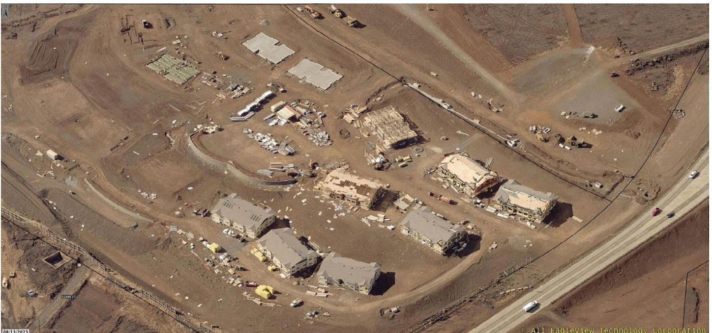
Figure 4.3.5.2.3 Wind damaged apartments at the construction site.
