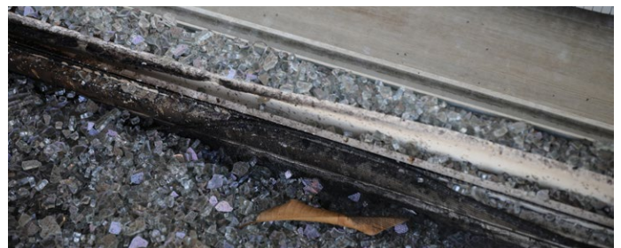
Figure 4.3.4.1.18 Destroyed chair proximate to rear patio door/window assembly on 4 Front Street, where the outer pane failed and inner pane remained intact. Note the indications of tempered glass in this assembly.
