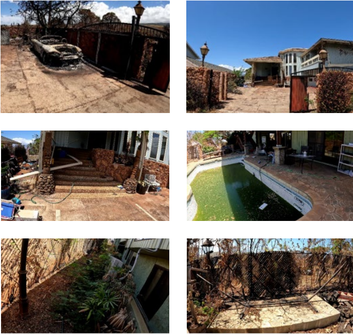
Figure 4.3.5.3.13 The 15███ Lokia Street lot experienced fire damage to the front entrance gate and destroyed a vehicle, but did not extend to the structure (top). The structure appears to have been defended, in part, by pumping water from the pool in the rear of the structure, powered by a battery system (middle). Damage to fences on the north and south sides of the properties (bottom), showing the end of the hose from the pump in the pool and along with a bucket (bottom left).
