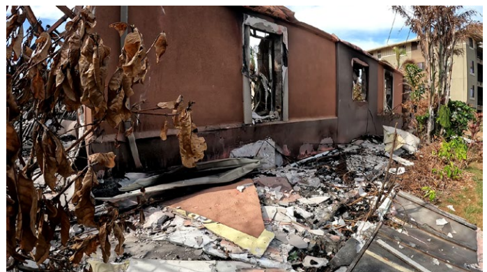
Figure 4.3.3.4.4 Destroyed apartment building showing CMU block exterior wall construction (first floor) and noncombustible sheathing with stucco finish coat and fiber cement siding.
