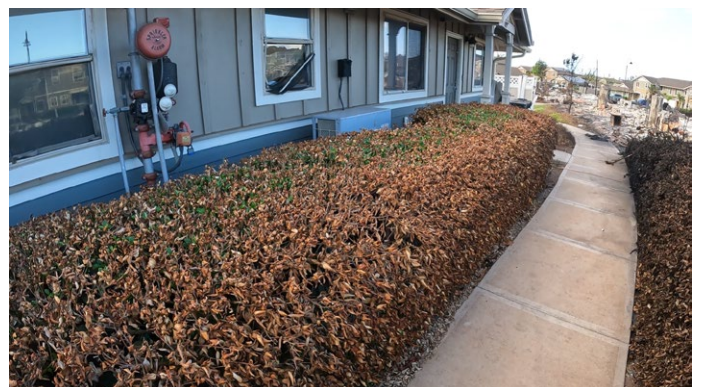
Figure 4.3.3.5.8 Ground-based photograph of space between Building 13 (shown on the left of the image) and Building 14 (shown on the right), showing damaged windows and heat damaged/dried (but not ignited) vegetation.
