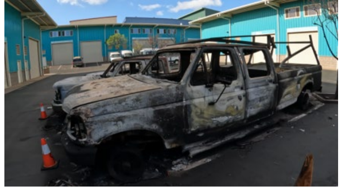
Figure 4.3.5.1.18 Vehicles consumed by fire in the middle of Emerald Plaza Place (near 1 █ Kupuohi Street).
