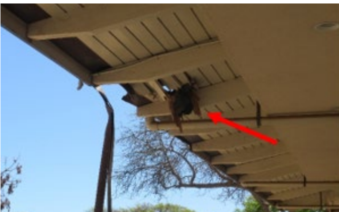
Figure 4.3.4.1.4 Utility pole south of Mill Street that hit and damaged the roof of the Boys & Girls Clubs of Maui.
