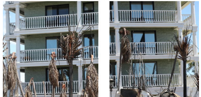
Figure 4.3.4.1.7 Increased window damage on the lower floor windows on the west-makai (right) compared to the east-mauka (left). Cracking is noted on the second and fourth floor windows with screens partially dropped on the third and fourth floors for the rooms on the west (makai).
