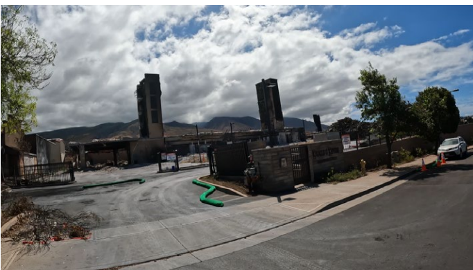
Figure 4.3.5.1.22 Kaiāulu o Kupuohi Apartment complex consumed by fire.
