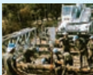
The SDF's first international peace cooperation activity in Cambodia. The SDF conducted road and bridge repairs, ceasefire monitoring, and other activities.
