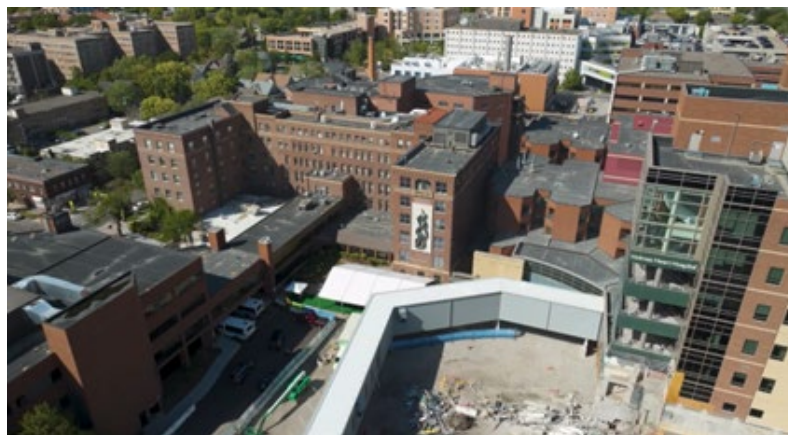
Construction is underway at Abbott Northwestern Hospital for a new surgical and critical care services building on the campus in south Minneapolis.
