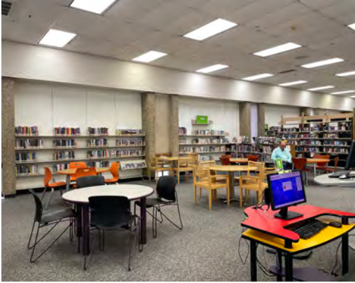
Park Forest Branch was assessed to be in “fair” condition in the 2018 Facility Condition Assessments.
