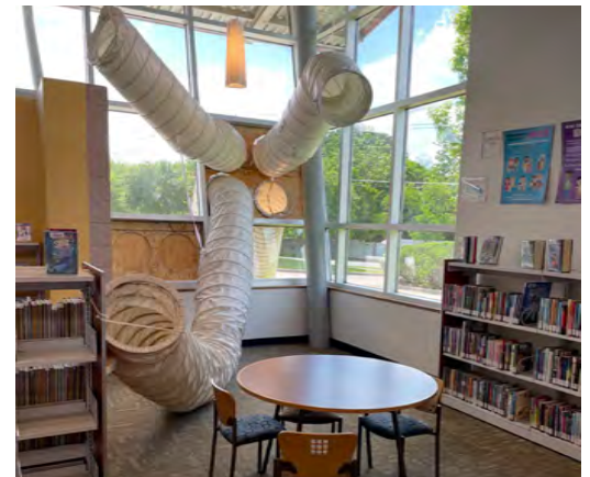
Temporary ventilation at Pleasant Grove Branch while its HVAC system waits for repair.
