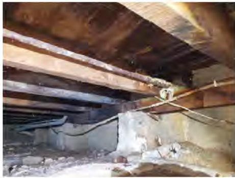
Image shows highly contaminated crawl space. Thermal insulation on the floor.
