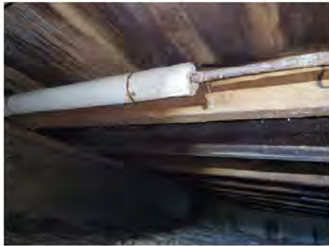
Image shows highly contaminated crawl space. Thermal insulation remaining on the pipes.
