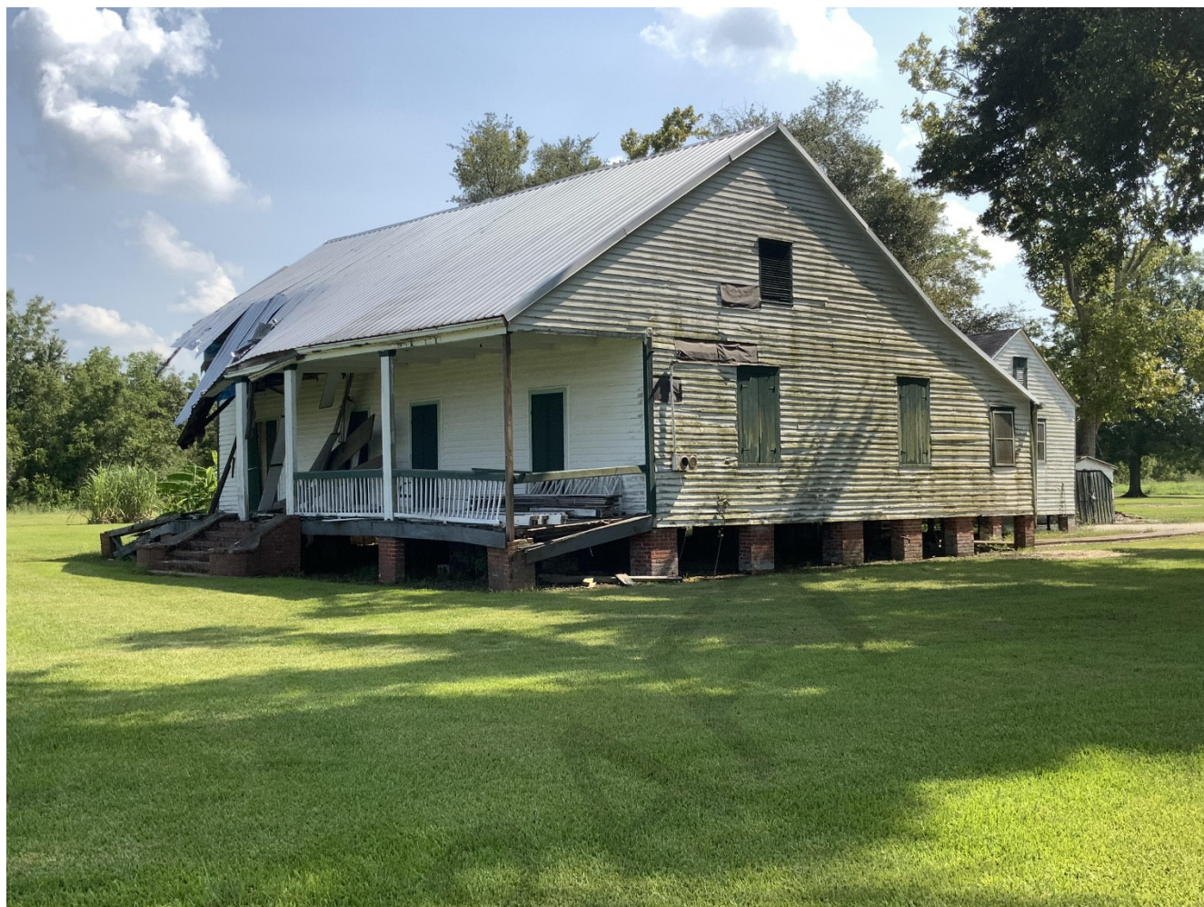
1 2 3 Figure 3-51. Photo of the creole cottage at 791 Highway 18 (ID#, 1465PIDN 0100049300). The Louisiana Trust has secured a grant to make repairs to the building. Source: Photo by HHM, 2023
