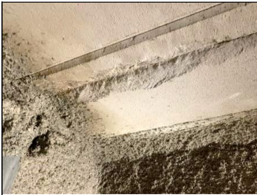
Photograph 6 Roof Area A2 – Spalling and exposed reinforcing bars
