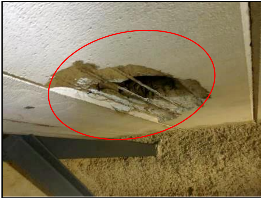
Photograph 7 Roof area A2 – Unreinforced field modification
