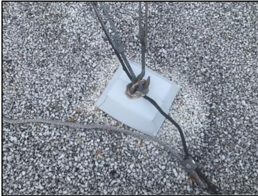
Photograph 19 Repair Area A1 - Sealant deficiency at stack supports
