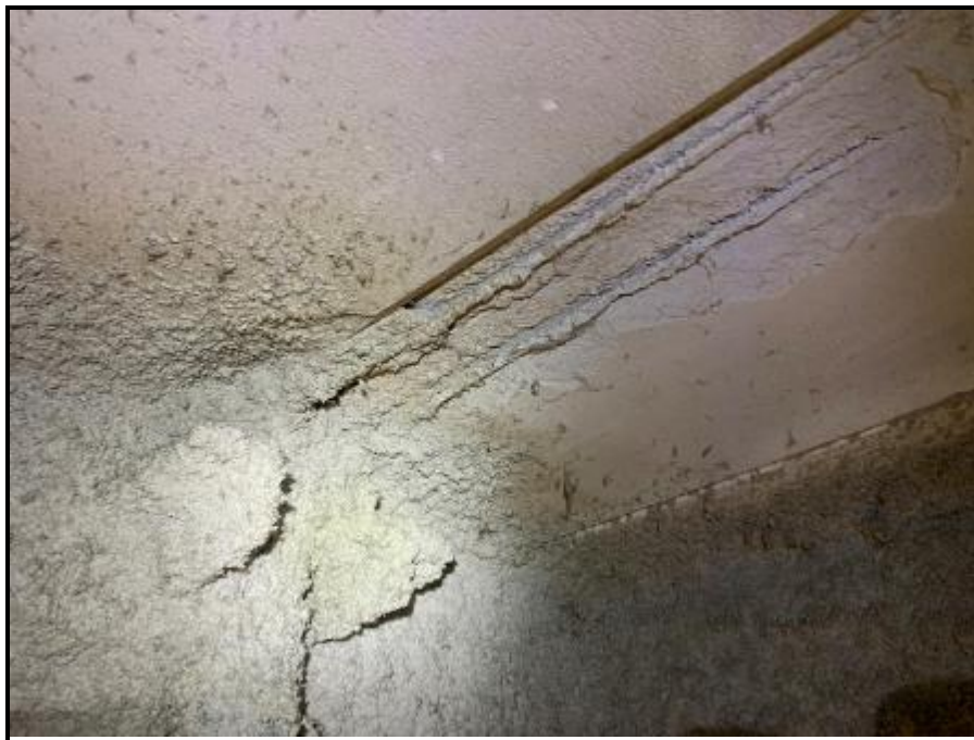
Photograph 2 Repair Location A1.1 – Spalling and exposed reinforcing bars
