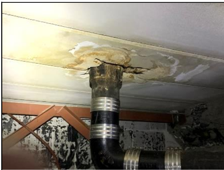
Photograph 8 Roof Area A2 – Excessive water staining and field modification
