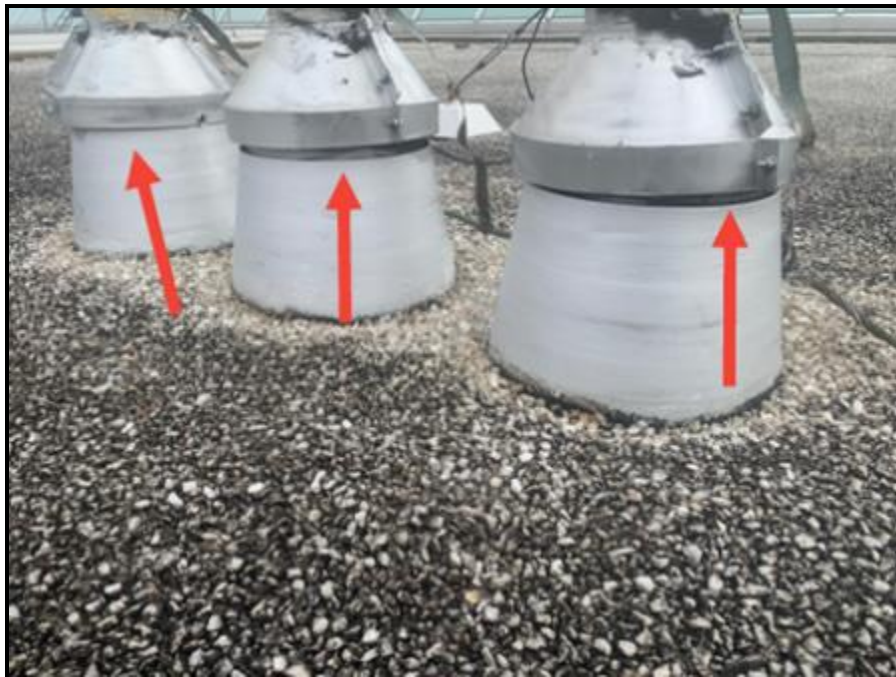
Photograph 20 Repair Area A1 - Opening at the top of the spun aluminum tall cones
