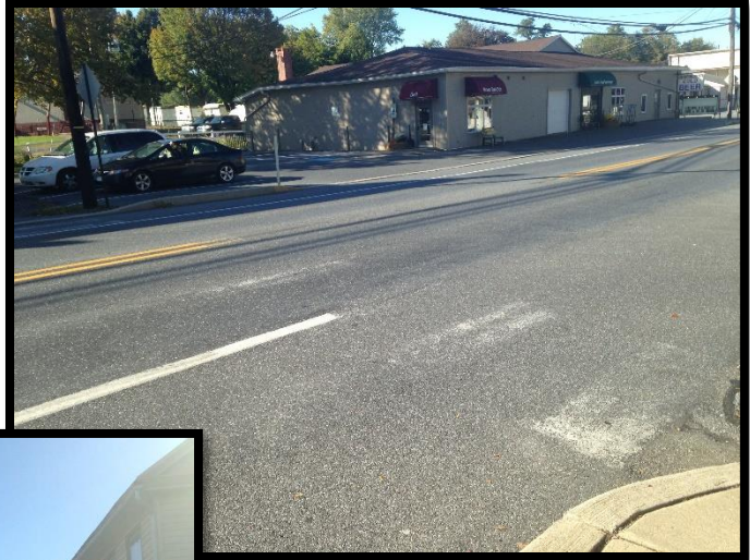
Figure 3: Faded Pavement Markings
