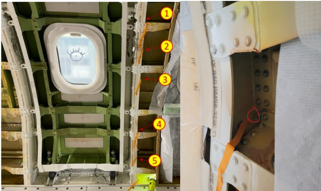
Figure 14. Photo on the left shows the five locations of the damaged rivets. Photo on the right is a close-up of a damaged rivet. (Source: Boeing. Image Copyright © Boeing. Reproduced with permission.)
