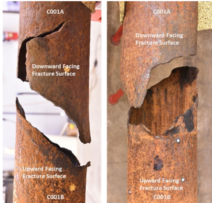
Figure 26: Photo of Axial Rupture and Parting of Joint C001 Rotated Approximately 180°
