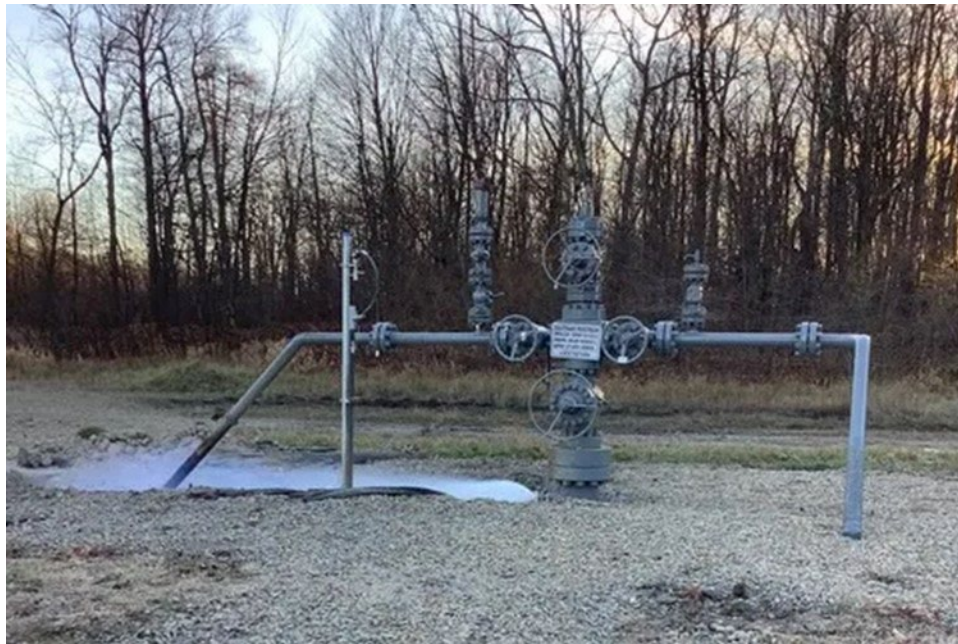
Figure 1: Well #2244 (George L. Reade #1) Gas Leaking Through the Annulus Valve
