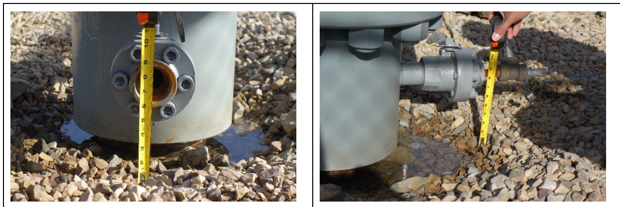
Figure 159: Well #2254, Annulus Valve Height Measurements, March 25, 2023, Open Side (Left) and Pressure Fitting Side (Right)
