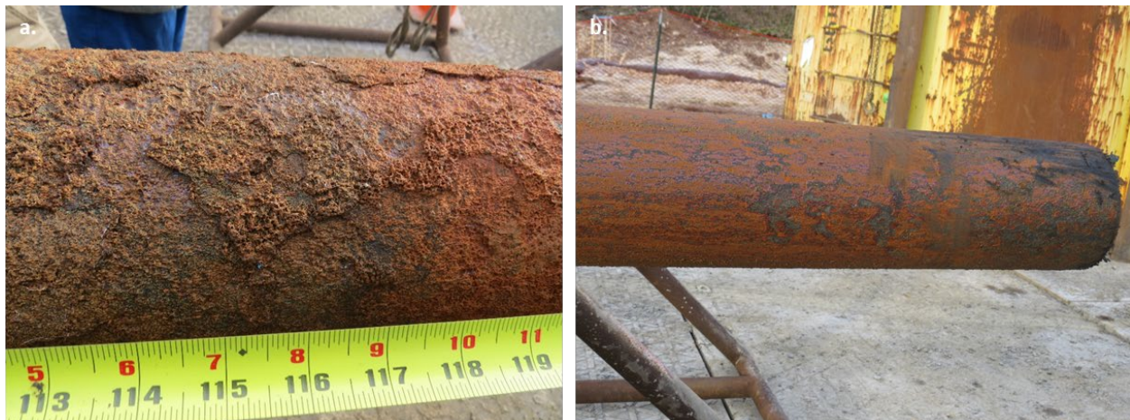
Figure 134: #2244 Joint C001B a. Top Portion Covered with Thick Scale, b. Bottom of C001B Cut End
