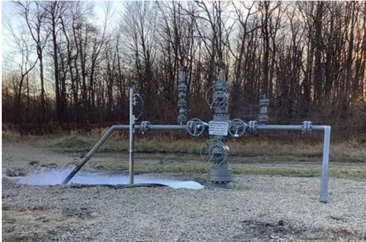
Figure 12: Well #2244 Venting Gas Out the Annulus Valve
