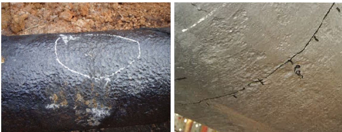
Figure 127: General Corrosion Observed in the Oil and Gas Industry
