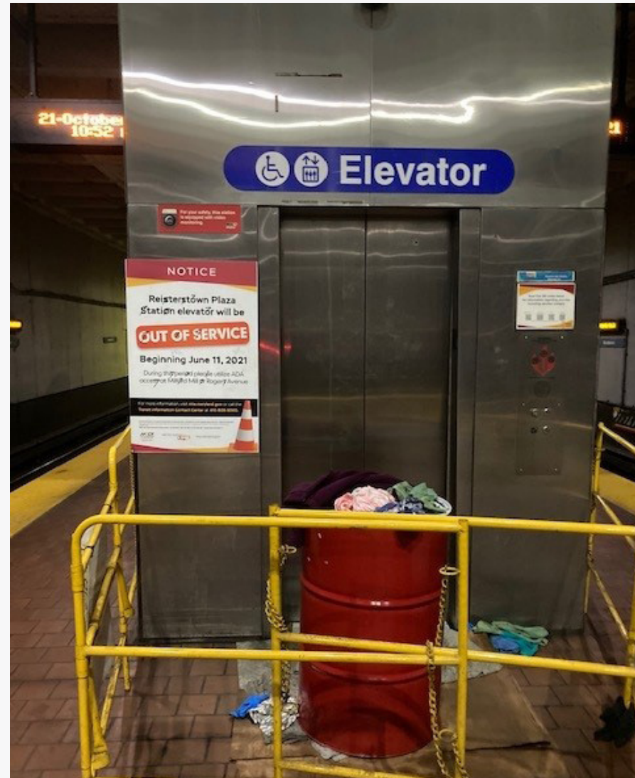
In 2022, MTA shut down both elevators (interior and exterior) at the Mondawmin Metro station, the agency's major transit hub in West Baltimore, for 18 months.
