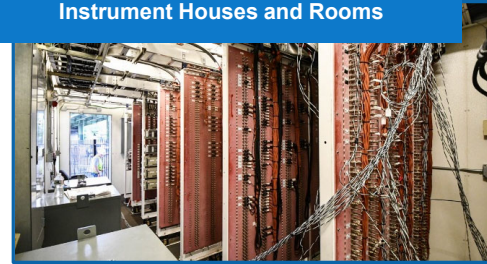
Instrument Houses and Rooms
