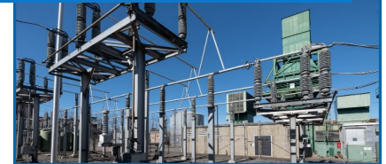
High Voltage Yard
