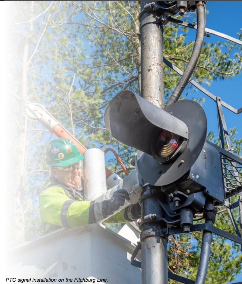
PTC signal installation on the Fitchburg Line.
