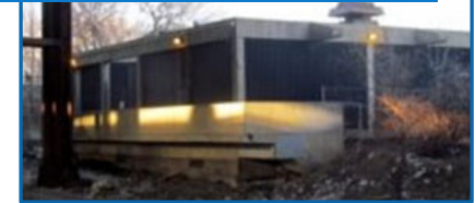
Unit Substation (USS) Equipment
