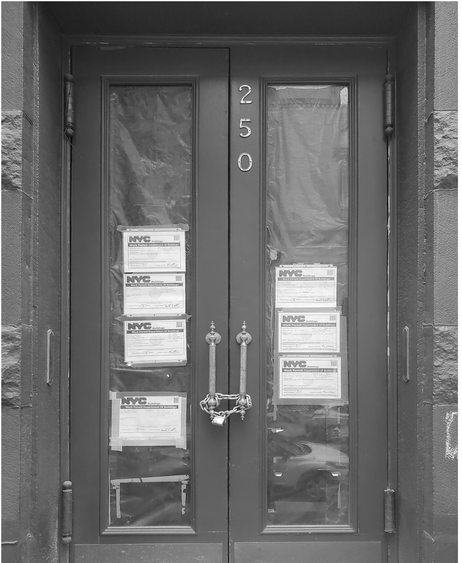
250 West 73rd Street mid-conversion This is the third row house to be converted from an apartment building to a single family home on the street where I live
