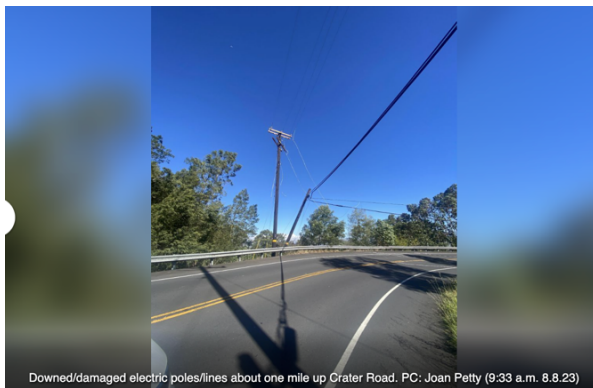
Downed/damaged electric poles/lines about one mile up Crater Road. PC: Joan Petty (9:33 a.m. 8.8.23)
