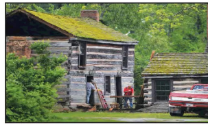
Workers begin to dismantle the historic Gilliland cabins in Charleston. AP file photo
