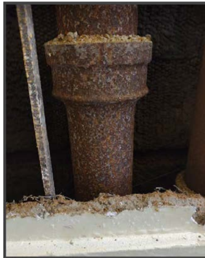
Waste riser at Howard considered to be in poor condition based on exterior physical appearance (excessive exterior corrosion)
