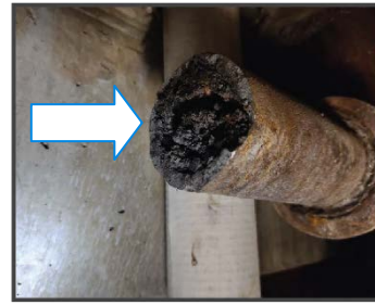
Interior surface of waste branch line (cast iron section) at Howard with significant sediment/debris accumulation
