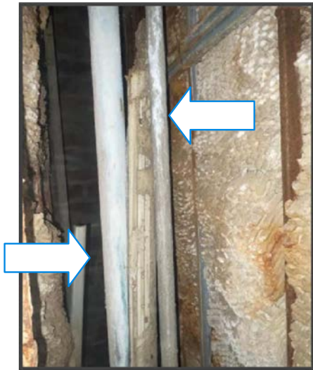
Domestic water risers at Queensbridge North displaying possible chemical reaction or de-zincification of the brass, suggesting that the pipes are at the end of their service life and may be subject to failure in the near term
