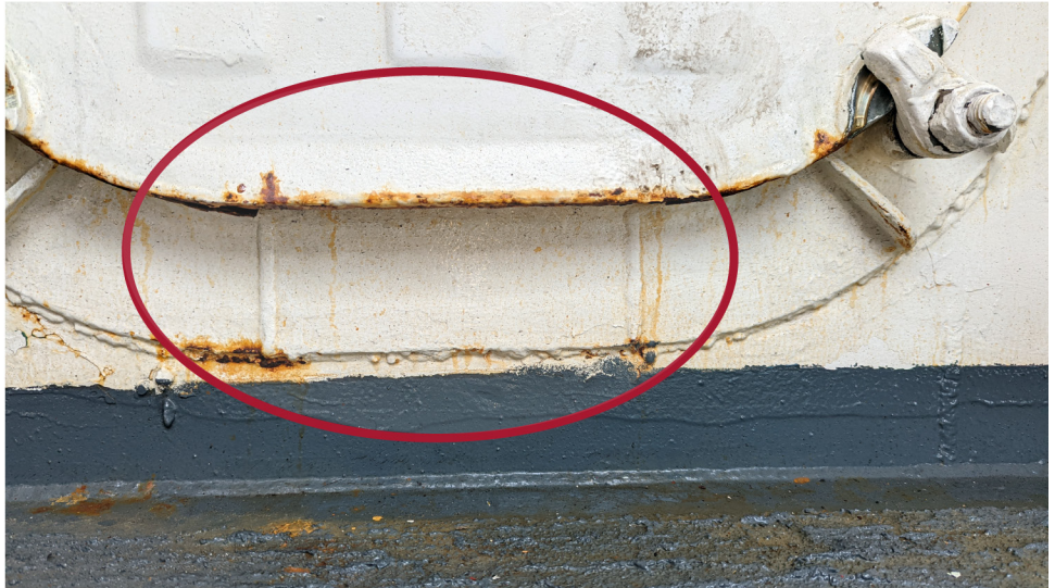
Figure 15: Rust on Exterior Door on 210-foot Medium Endurance Cutter (MEC)
