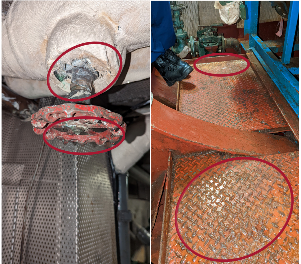
Figure 14: Condensation on Piping (left) and Corrosion on Slippery Surface (right) on 210-foot Medium Endurance Cutter (MEC)
