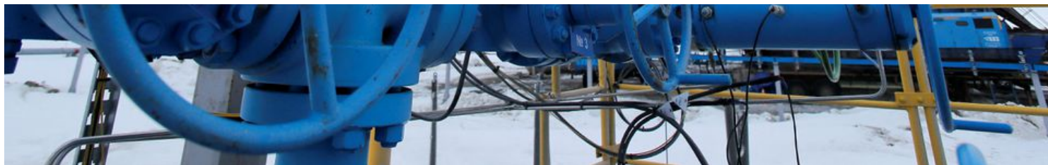
A view shows valves near a drilling rig at a gas processing facility, operated by Gazprom company, at Bovanenkovo gas field on the Arctic Yamal peninsula, Russia May 21, 2019. Picture taken May 21, 2019. REUTERS/Maxim Shemetov/File Photo
