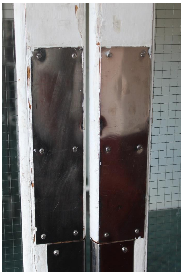
Photo 13: Close-up of smoke-stop doors
