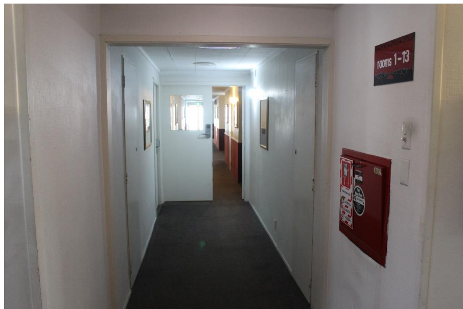
Photo 5: A Block - Firehose reel
