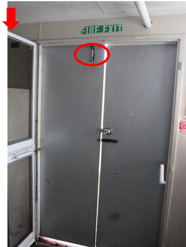
Photo 18: A Block – Fire exit door, ground level
