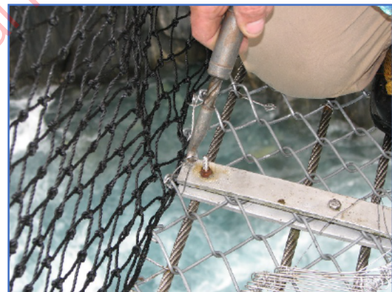
Fig. 7 Re-fixing barrier in-fill netting with wire loop ties.
