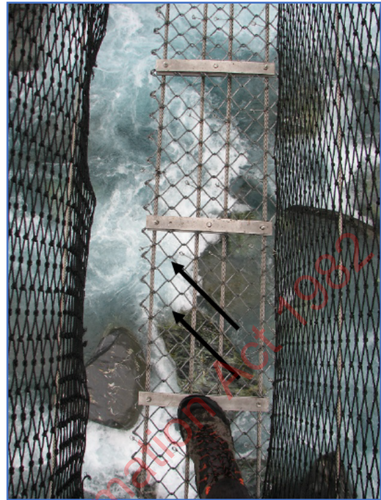
Fig. 6 Detached barrier-infill netting where the fall occurred. Arrows show 'slip-direction' of chain link netting.
