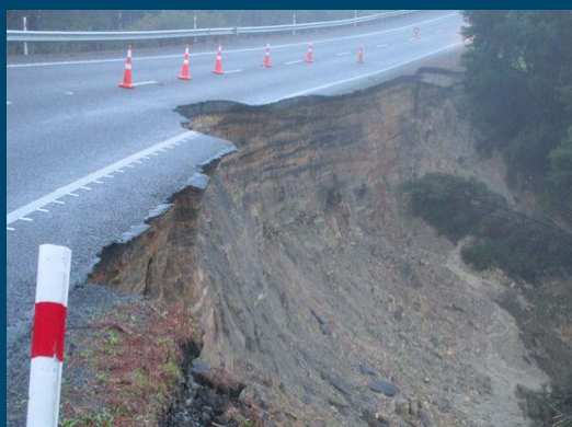
Left: State Highway 1 at Maromaku, south of Kawakawa, remains closed due to storm damage.
