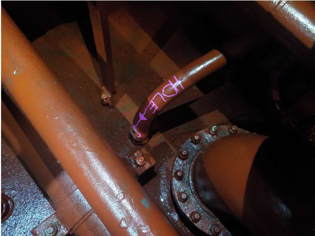
Figure 1: Hole in Vent Header to Tank (b) (3) (A)
