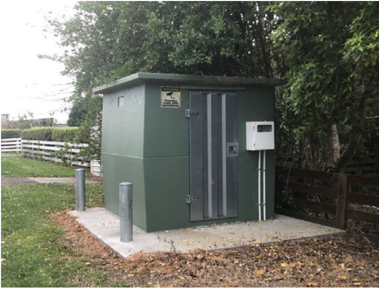
Figure 9 Fraser Street Booster Pump Station
