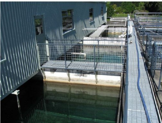
Figure 7 Gravity sand filters
