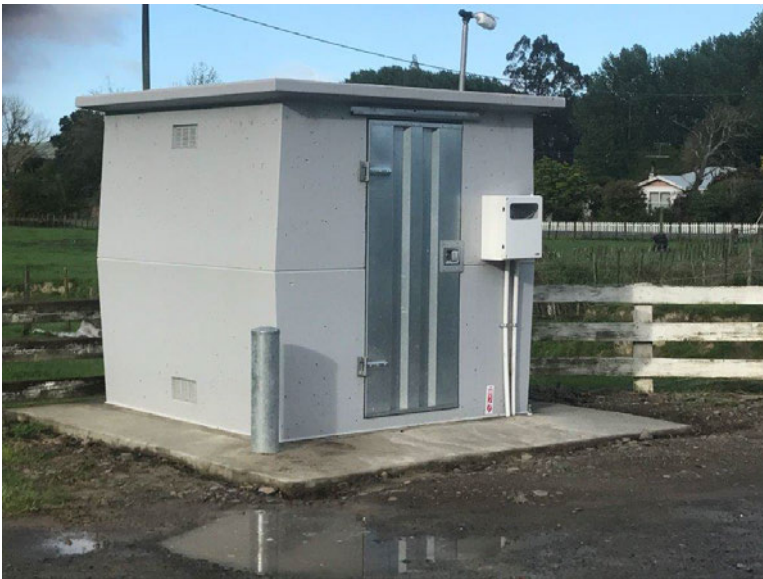
Figure 10 Awatere Booster Pump Station
