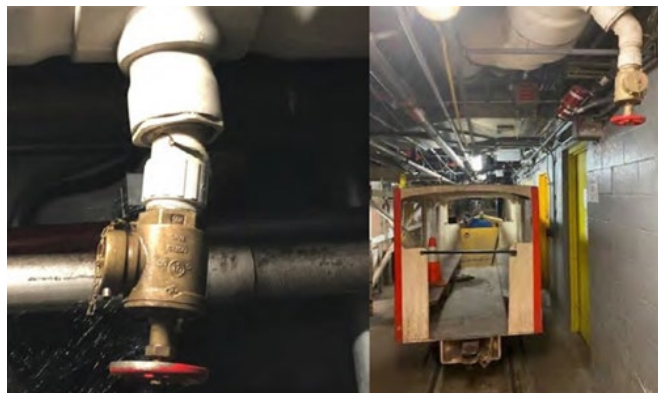
Cracked Low Point Drain
