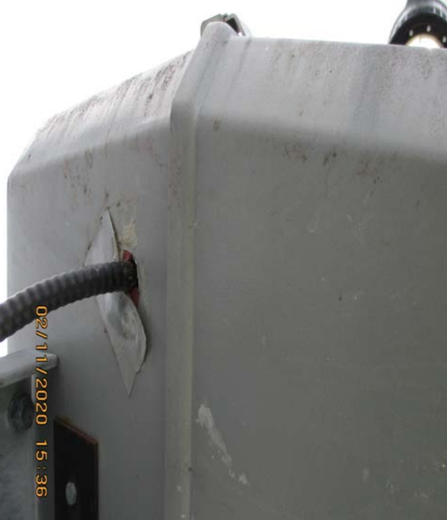
Duct Tape is used to seal this off from a Class 1 Division 2 classified area instead of a proper sealant. AKOSH Inspection Report 1449721.015.
