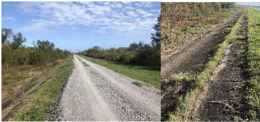
Figure 35a. Crest of river levee fronting LNG site and 35b. river side shown crack concrete capping.
