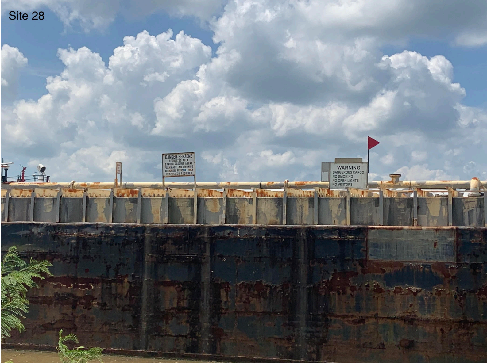
Figure 12: A closer look at site 28 in Reserve, LA where a benzene warning sign is clearly visible. Benzene is a known human carcinogen. There is a community located right on the other side of the levee where this photo was taken.
